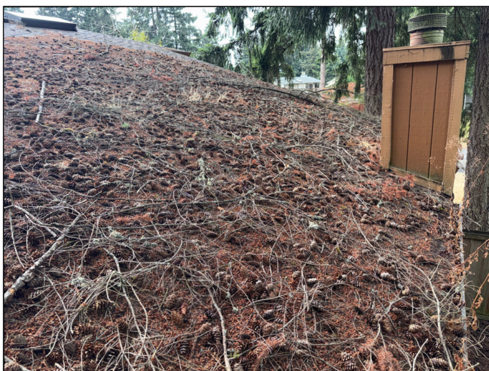
Debris on Roof
