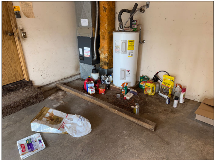
Recommend repairing the wood curb to ensure a vehicle does not hit the furnace or water heater.
