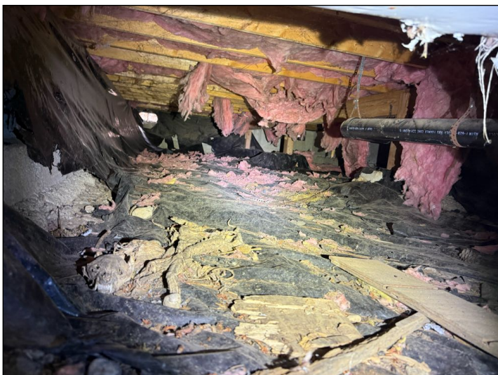
Rodent droppings present in the crawlspace. Recommend monitoring for activity and repair as needed.
