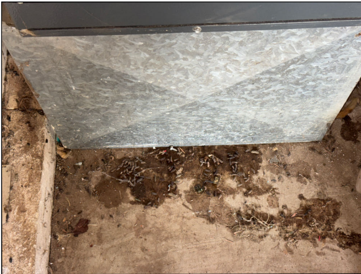
Rodent droppings noted on the concrete floor around the furnace in the garage.
