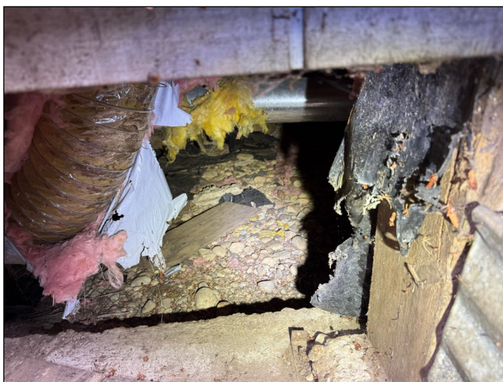
Debris and fallen insulation were noted throughout the crawlspace. These materials can provide nesting areas for rodents and create conditions conducive to wood-destroying organisms. Recommend removing all debris and damaged insulation. Install new vapor barrier as needed.
