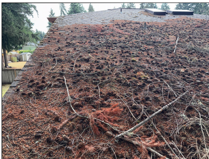
Debris on Roof
