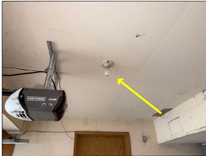
One the garage lights not functioning.
