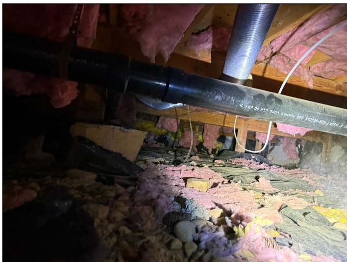
Debris and fallen insulation were noted throughout the crawlspace. These materials can provide nesting areas for rodents and create conditions conducive to wood-destroying organisms. Recommend removing all debris and damaged insulation. Install new vapor barrier as needed.
