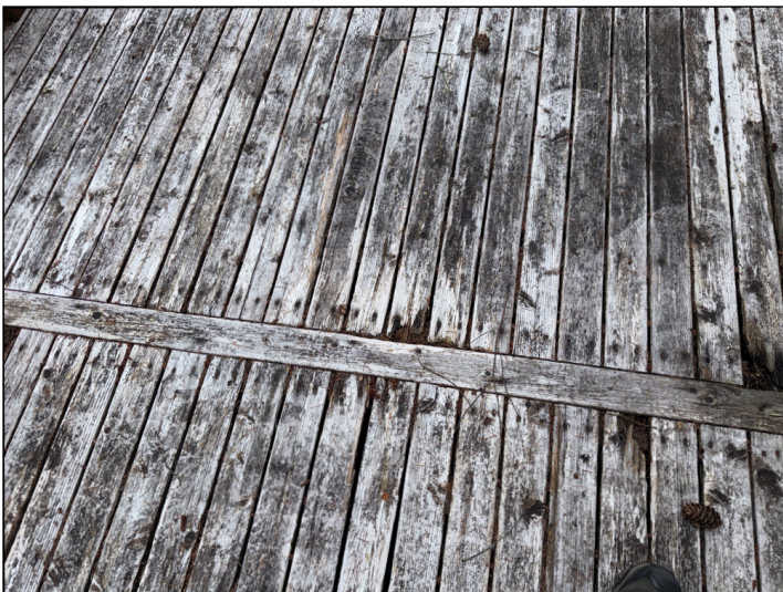
Some boards at the deck were rotting/deteriorating. Recommend replacing damaged boards as needed.
