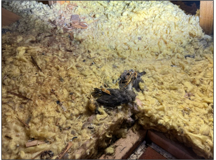
Multiple bird nests and entry points were noted on the south side of the attic. Bird nesting materials, droppings, and dead birds were observed throughout the attic insulation. Recommend professional removal and cleaning, replacement of contaminated insulation as needed, and sealing all entry points to prevent future access.
