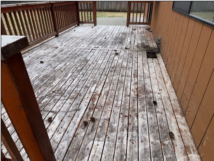
The wood deck is in poor condition and should be budgeted for replacement.
