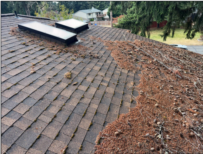
Debris on Roof
