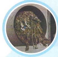
Wipes can cause breakdown of pumps in pump stations.
