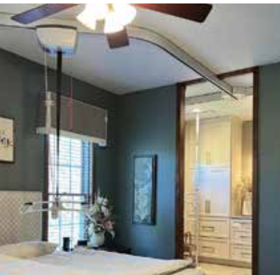
Amy Buren's (LGMD R1/2A) ceiling lift with track system is permanently installed on the ceiling.
