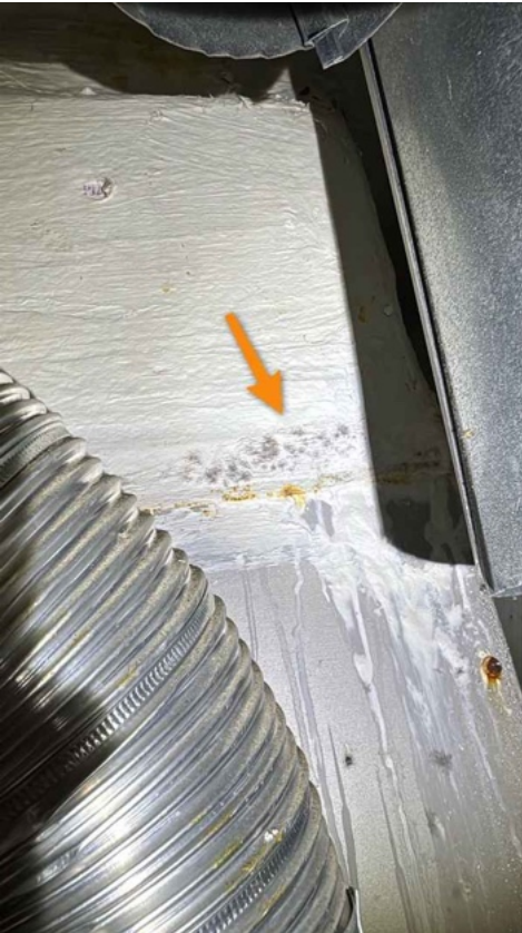
On HVAC unit
