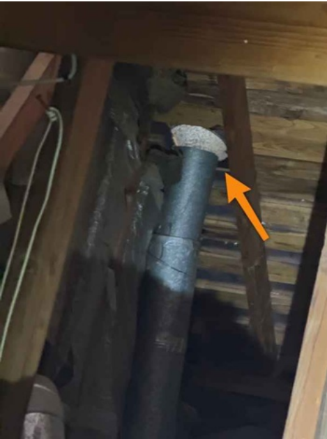
Range hood not sealed through the roof
