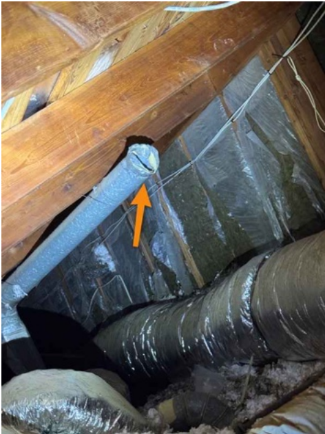
Dryer vent terminates to attic
