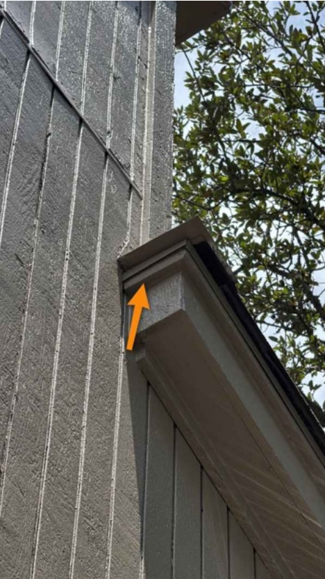
Left side of home. Ridge cap flashing not properly installed. Water can get underneath.
