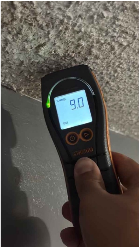
Garage Ceiling Stain
