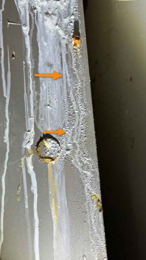
Excessive condensation on HVAC unit
