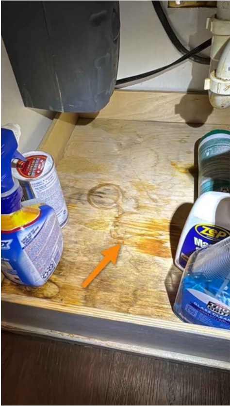
Clean under kitchen sink
