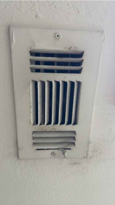
Dirty supply grill. Laundry Room
