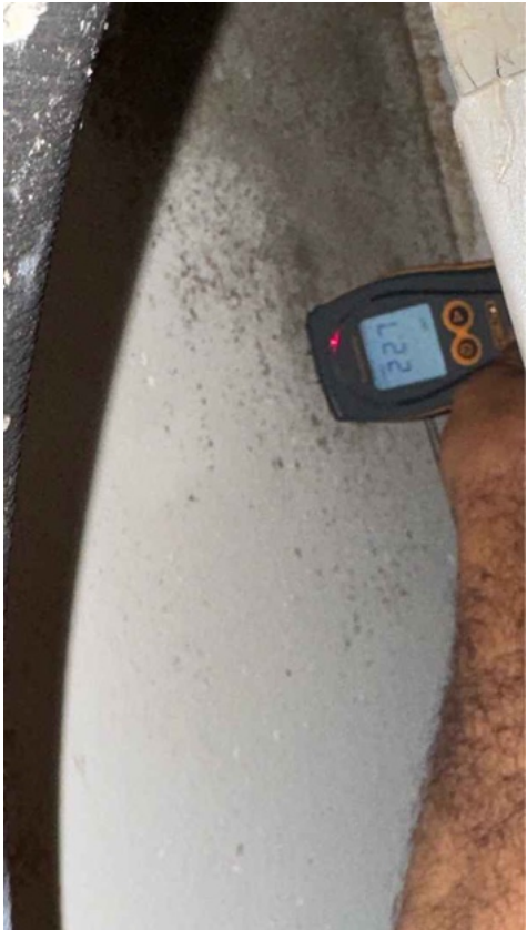
HVAC Closet wall. Elevated moisture reading.
