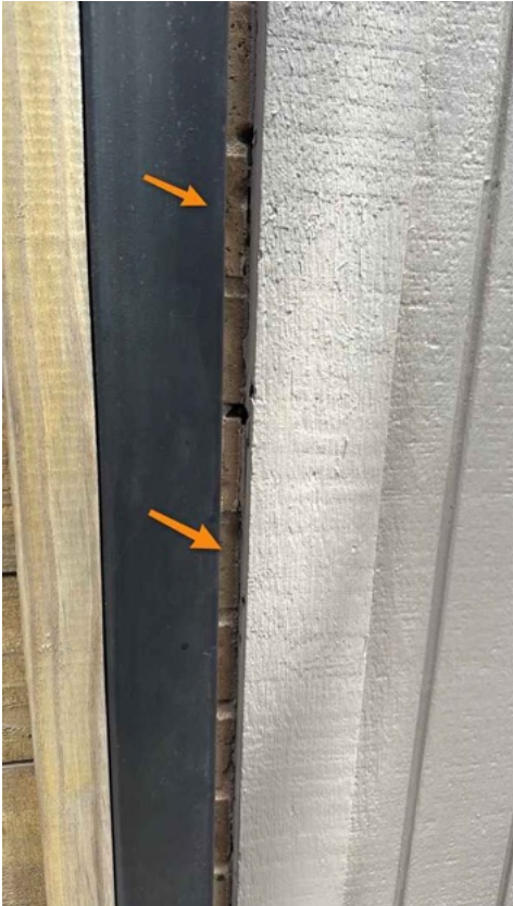
Back Right Corner Of Home. Add exterior sealant
