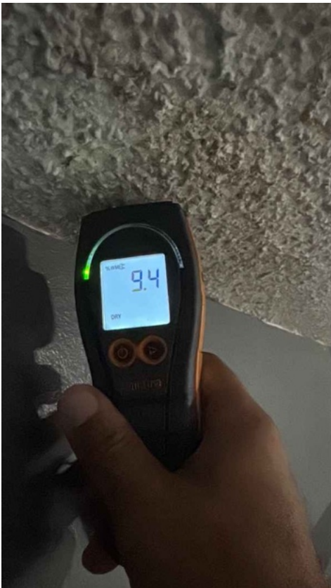
Garage Ceiling Stain
