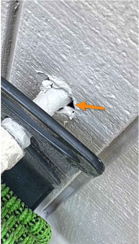
Right Side Of Home. Exterior sealant needed.
