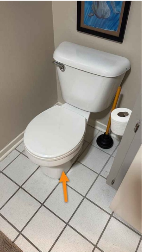
Hallway Bathroom. Loose toilet
