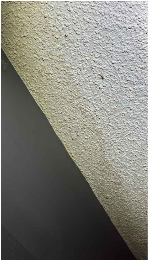
Garage Ceiling Stain
