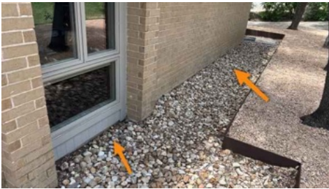
Front Of Home. Negative grade and soil line too high.
