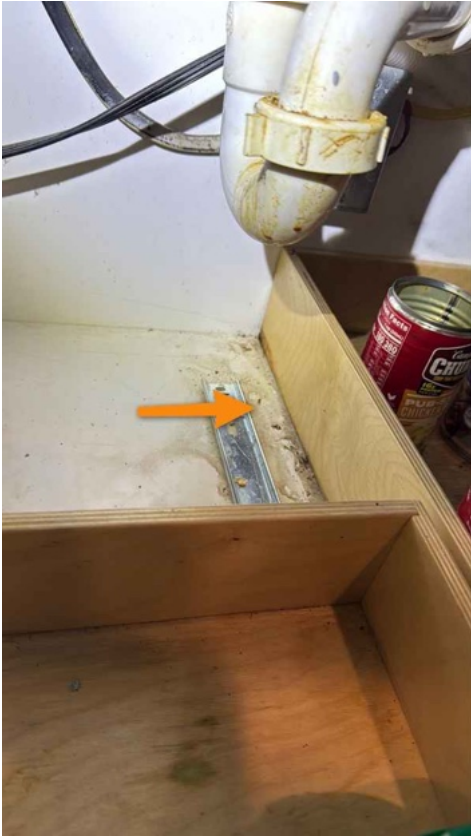
Clean under kitchen sink
