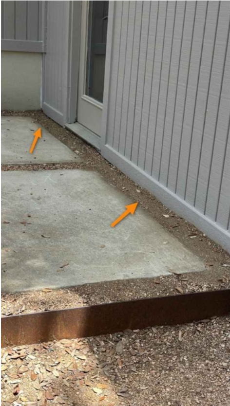
Right Side Of Home. High soil lines.
