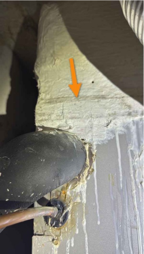
Excessive condensation at HVAC refrigerant line penetration
