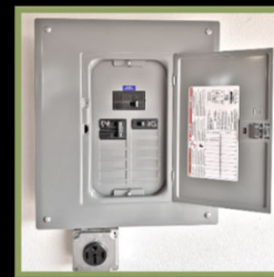
Garage Metering & Wiring
