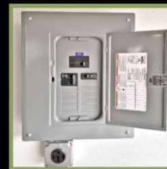
Garage Metering & Wiring
