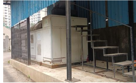
OWC MACHINE ON SITE
