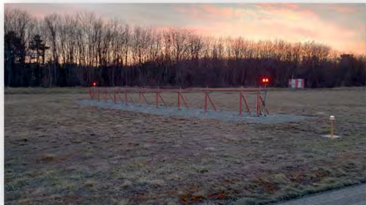
Figure 2-9 End Fire Glideslope Runway 14 End
