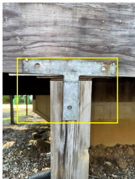
Questionable deck construction
