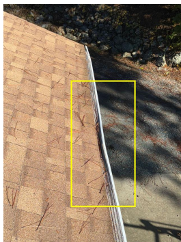
Damaged front gutter
