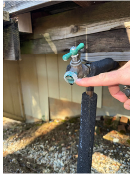
Leaking left side hose bibb
