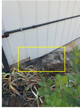
Siding to ground contact
