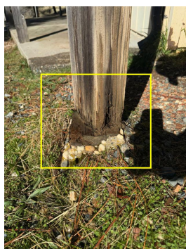
Decayed deck post
