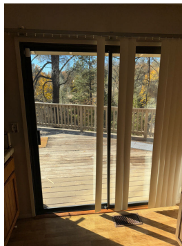
Missing sliding screen door
