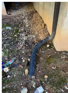
Drainage system not inspected
