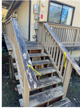
Handrails not graspable
