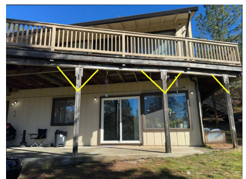
No deck lateral bracing
