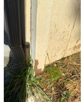
Deficient paint on siding
