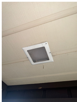
Light fixture inoperable
