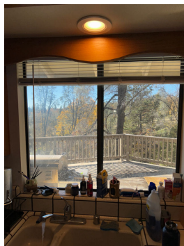
Failed window seal
