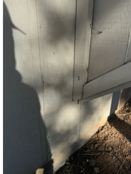
Deficient paint on siding
