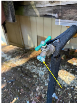
Missing anti siphon vacuum breaker
