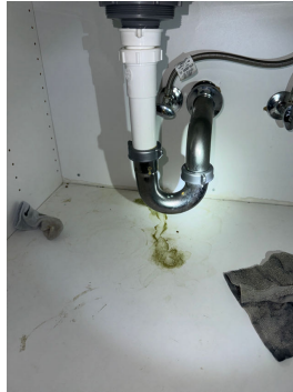
Metal sink trap with evidence of leaking
