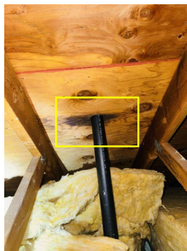
Attic leak stain
