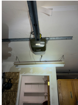
Light fixture inoperable
