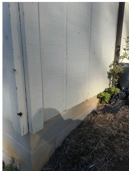
Deficient paint on siding
