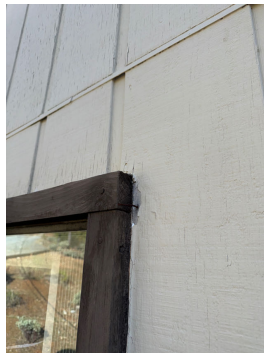
Deficient paint on siding
