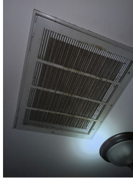
Dirty HVAC filter
