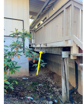
Sagging deck beam
