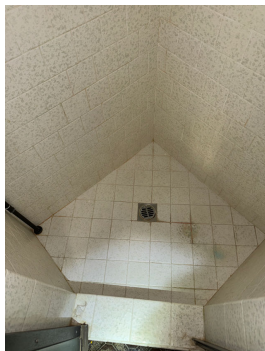
Stained and discolored shower pan
