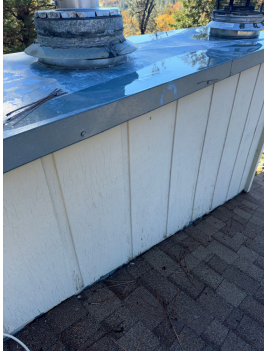
Deficient paint on chimney
