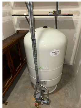
Pressure tank detail
