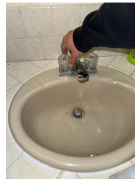
Deficient sink stopper
