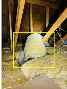
Torn vapor barrier on ductwork
