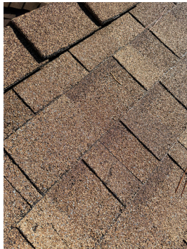
Light roof wearing
