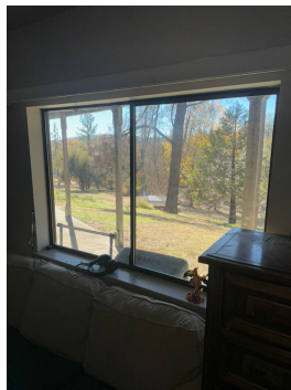
Missing downstairs bedroom screen
