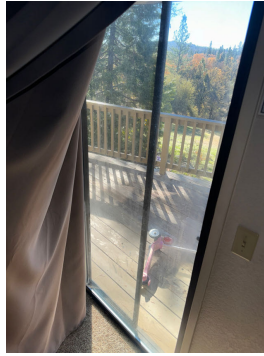
Failed door glass seal
