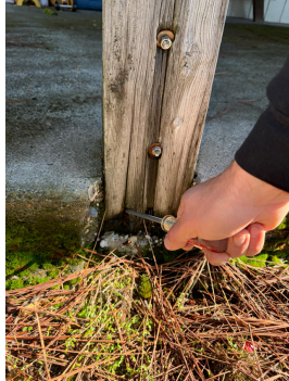
Decayed deck post
