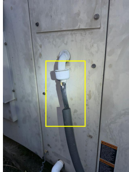
Loose conduit with exposed wiring
