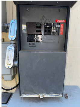
Main breaker box detail
