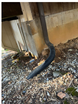
Drainage system not inspected
