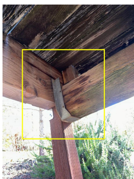
Questionable deck construction
