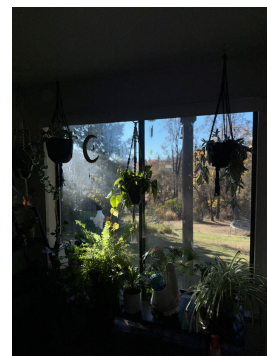
Failed downstairs window seal
