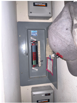
Main panel detail
