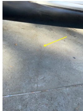
Minor driveway crack
