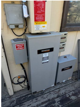
Auxiliary generator system not inspected
