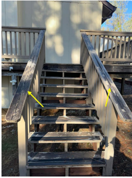
Handrails not graspable
