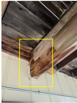
Questionable deck construction
