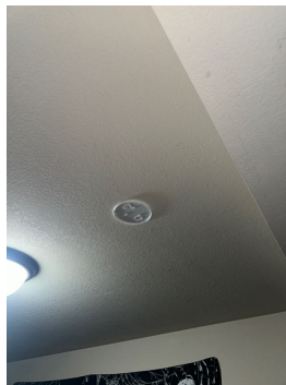
Missing downstairs bedroom smoke alarm
