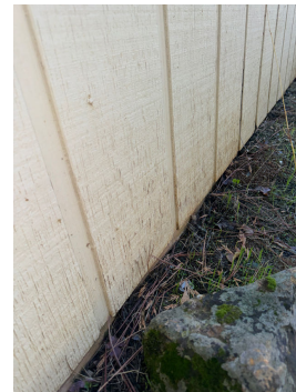
Deficient paint on siding
