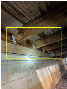
Ledger installed with nails and lacking flashing
