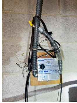
Pump system not inspected
