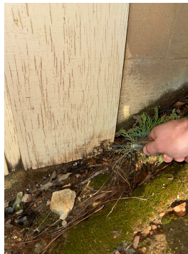
Left side siding to ground contact and decay
