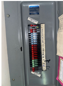
Zinsco brand circuit breakers
