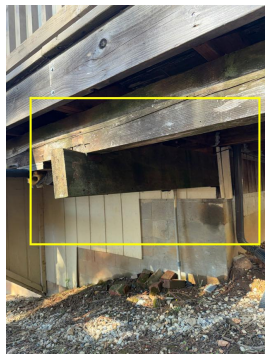
Questionable deck construction, sagging cantilevered beam
