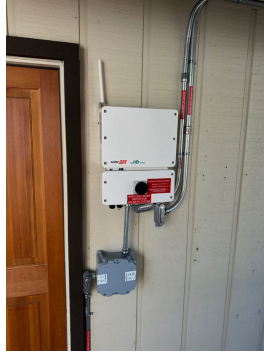
Solar array system not inspected
