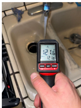
Water temperature noted at 121.6° F
