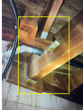
Questionable deck construction
