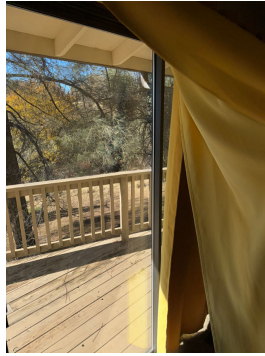
Bedroom 12 missing sliding screen door
