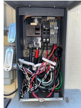
Main breaker box detail
