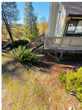
Negative grade toward house
