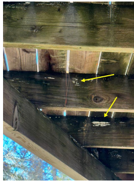
Fungal growth on underside of deck
