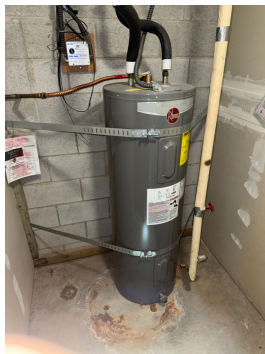
Water heater detail
