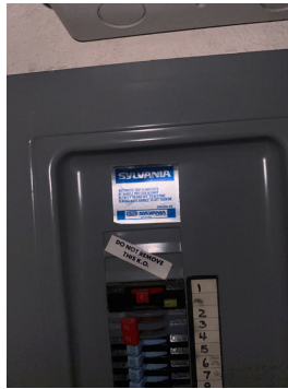
GTE Sylvania brand electrical panel
