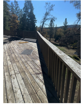
Railing height under 42"
