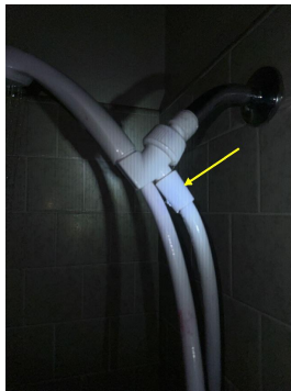
Leaking shower head
