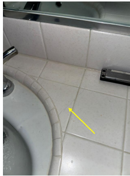
Bathroom 2 cracked tile
