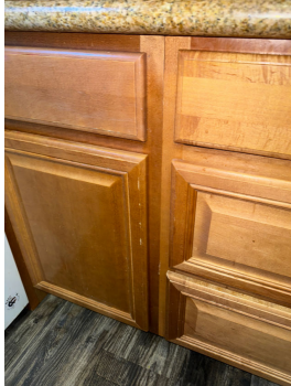
Worn cabinet finish
