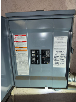
Sub panel detail
