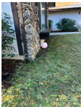
Negative grade toward house
