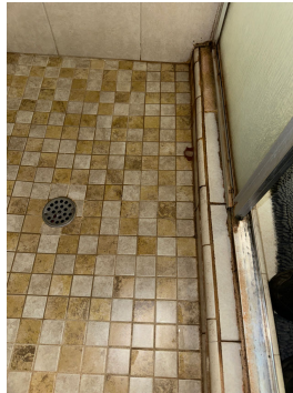
Bathroom 2 shower pan stain/discoloration
