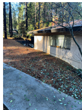
Negative grade toward house
