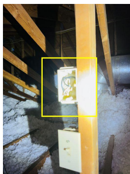
Open junction box
