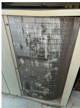
Damaged/bent cooling fins
