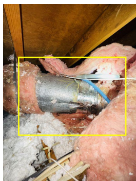
Deficient insulation on ductwork
