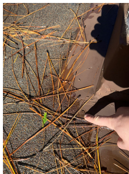
Unsealed flashing nail
