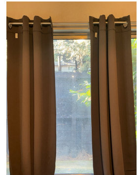
Bedroom 10 failed window seal
