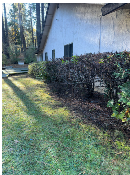
Negative grade toward house
