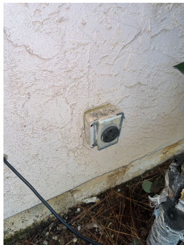
Back left corner missing waterproof cover
