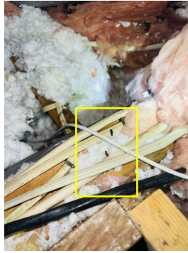
Rodent droppings in attic
