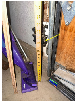
Photo electric sensor over 6" from ground
