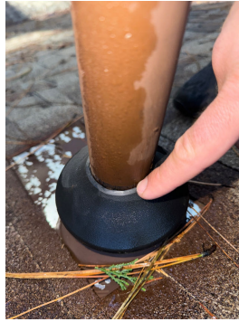
Worn/loose vent pipe rubber boot
