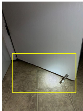
Damaged bathroom 1 door skin
