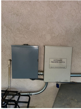
Auxiliary generator system not inspected
