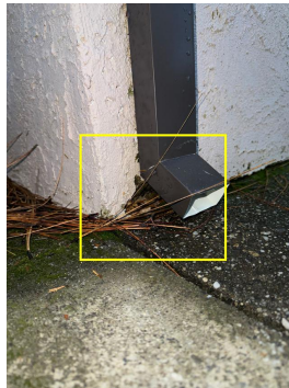
Back right corner stucco damage
