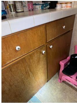
Worn bathroom 1 cabinets
