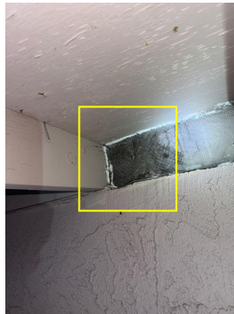
Exhaust duct terminates at soffit vent
