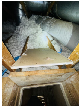
Uninsulated attic access hatch
