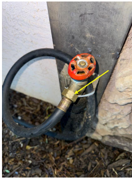
Missing anti siphon vacuum breaker
