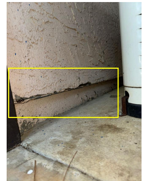
Front right corner damaged stucco
