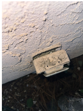
Back left corner elecrcial box loose on wall
