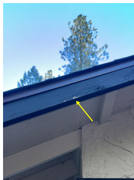
Deficient paint and/or caulk
