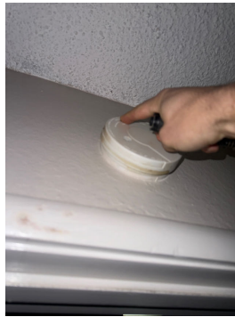
Bedroom 7 smoke alarm inoperable
