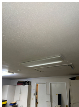
Light fixture inoperable
