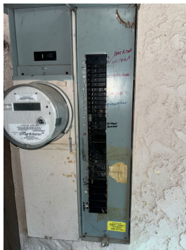
Main service panel detail
