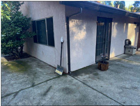
Stucco to patio contact
