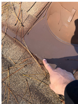
Unsealed flashing nail
