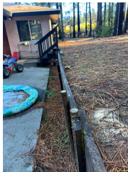
Leaning retaining wall
