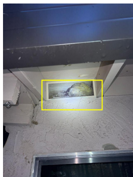
Soffit vent blocked with insulation
