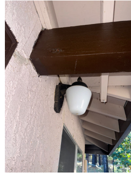
Light fixture inoperable
