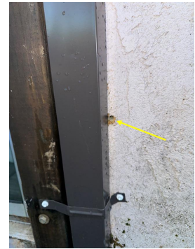
Back left stucco holes
