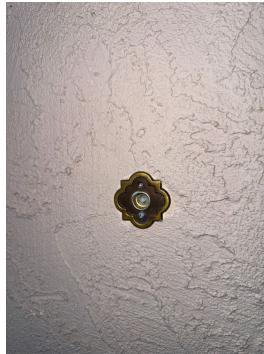
Damaged door bell button
