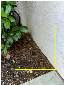
Right side stucco to soil contact
