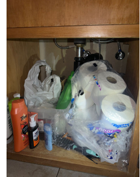
Blocked bathroom 2 cabinet
