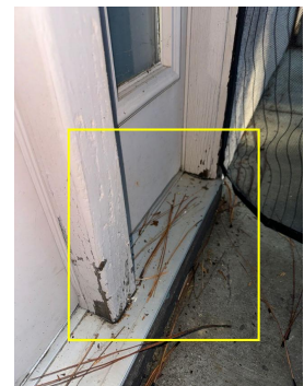
Deficient paint and/or caulk
