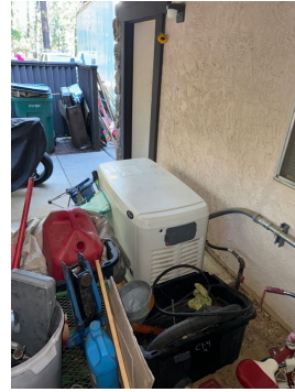
Auxiliary generator system not inspected
