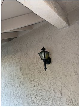
Light fixture inoperable
