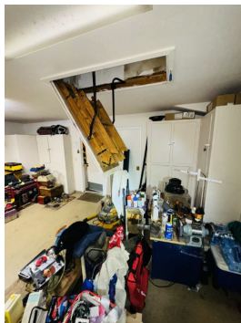
Blocked attic access hatch
