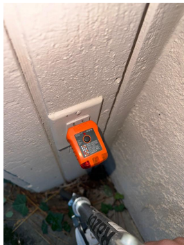
No power to outlet
