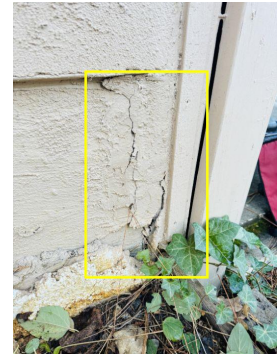
Back right foundation wall crack
