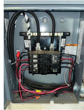
Sub panel detail
