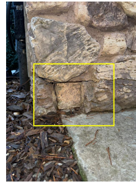
Missing masonry stone
