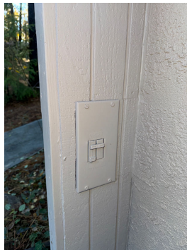
Missing waterproof box for panel
