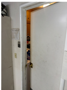
Deficient self closing device on fire door
