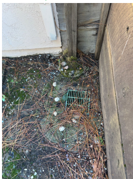
Drainage system not inspected
