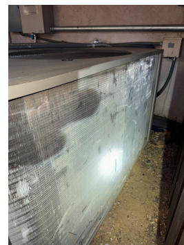
Damaged/bent cooling fins
