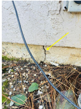
Back left foundation wall cold joint
