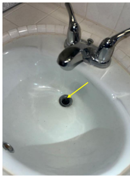
Missing bathroom 2 sink stopper
