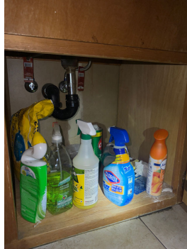
Blocked bathroom 2 cabinet
