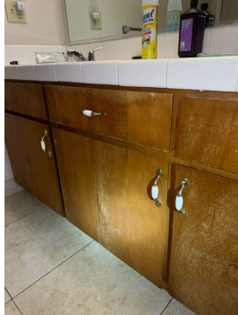
Worn bathroom 2 cabinet finish
