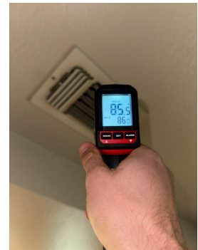
Inadequate heating temperature at 85.5° F
