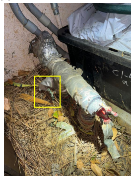
Secondary water shut off valve
