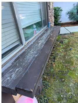
Deficient paint and/or caulk
