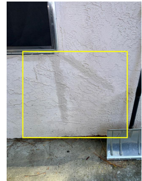
Patched stucco cracks, right side
