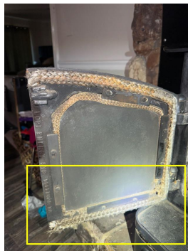
Damaged door rope gasket
