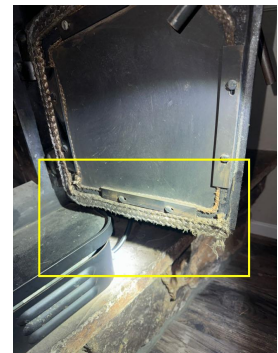
Damaged door rope gasket
