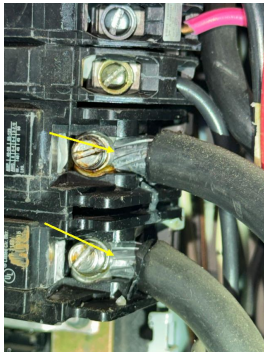
Missing anti oxidant paste
