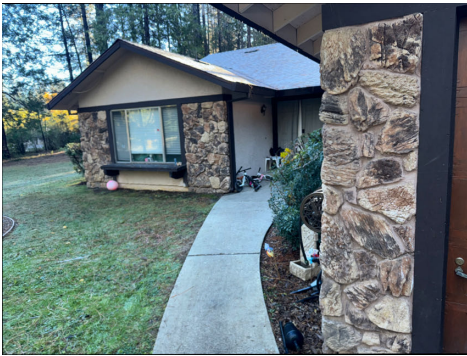
Masonry veneer lacking drain plane
