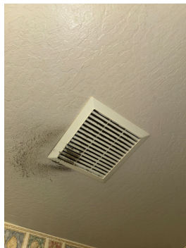
Clogged bathroom 1 exhaust vent
