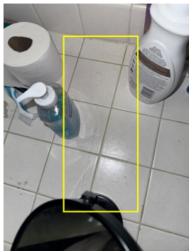
Bathroom 1 counter tile cracks
