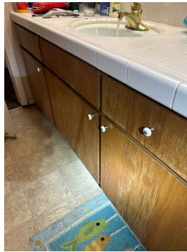
Worn bathroom 1 cabinets
