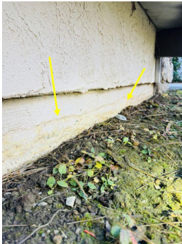
Foundation wall cold joint
