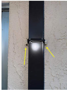
Back left stucco holes
