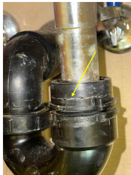
Bathroom 2 damaged drain pipe
