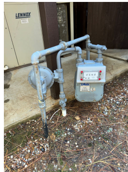
PG&amp;E gas meter and shut off valve
