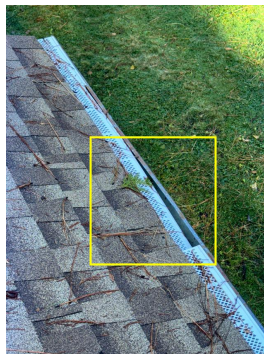
Damaged/out of place gutter screen
