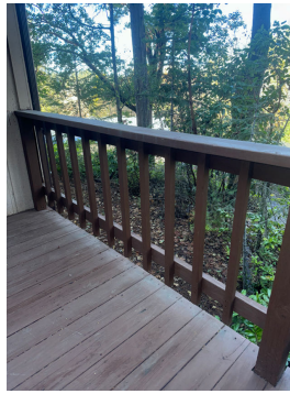
Baluster spacing over 4", height under 42"
