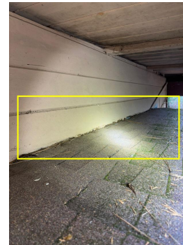
Siding to roof contact and wood decay
