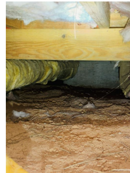
No access due to ducting
