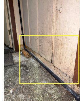
Back side siding decay
