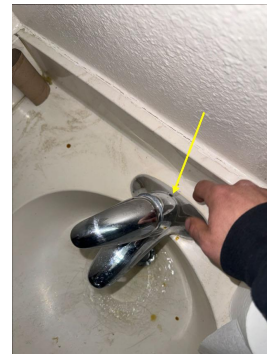
Bathroom 2 missing sink stopper handle
