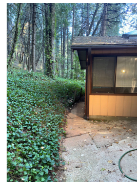
Negative grade toward house
