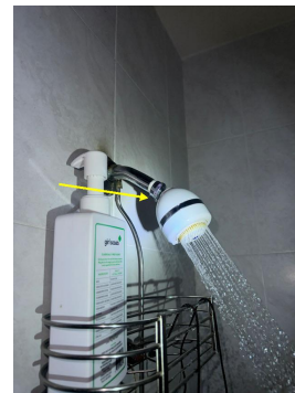
Bathroom 2 leaking shower head
