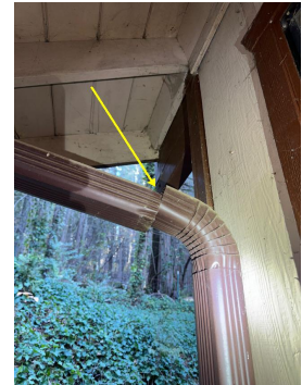
Disconnected back left downspout section
