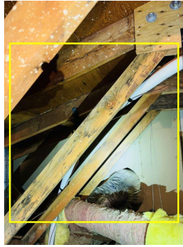
Black staining on attic structure
