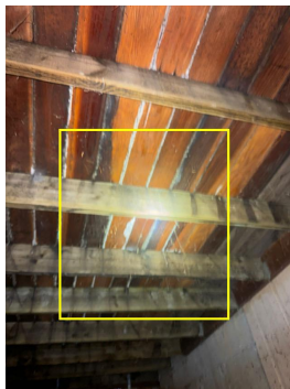
Fungal growth under deck
