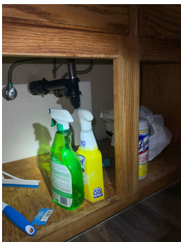
Bathroom 1 blocked sink cabinet
