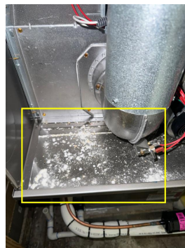
White powder/corrosion inside furnace cabinet
