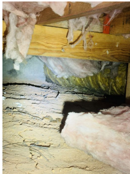
No access due to ducting
