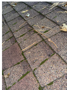
Moss on roof
