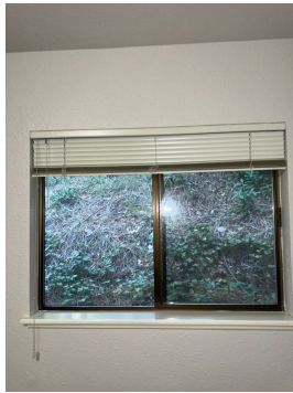
Room 5 possible failed seal
