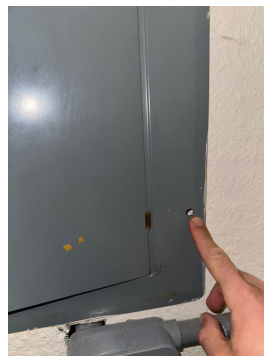
Missing panel cover screw
