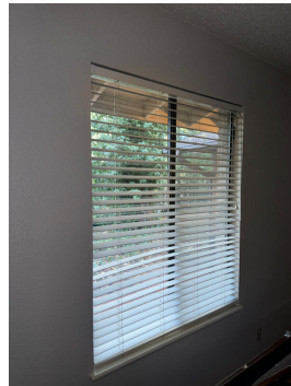
Entryway window difficult to open
