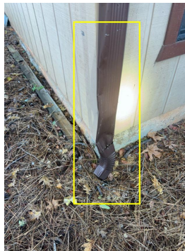
Downspout terminates at foundation and is damaged
