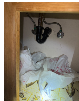
Bathroom 2 blocked sink cabinet
