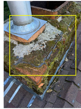
Cracked chimney crown
