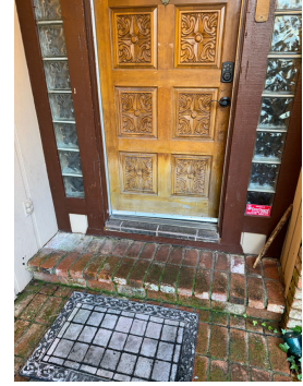
Front siding to ground contact
