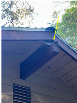
Decayed back side beam end
