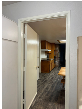
Deficient self closing device on fire door
