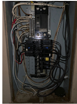
Main service panel detail
