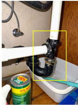
Evidence of past drain line leak
