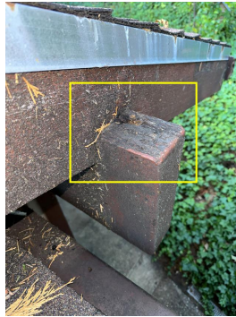
Decayed back side beam end
