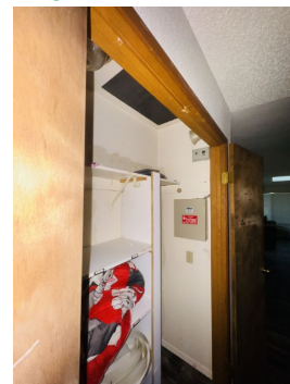
Blocked closet attic access
