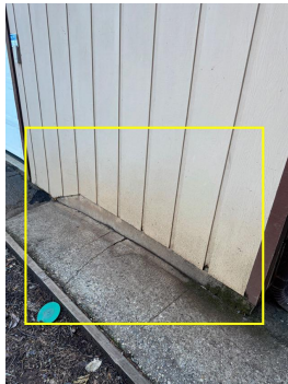
Back right side siding wood decay
