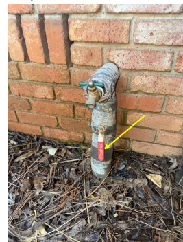
Possible secondary water shut off valve
