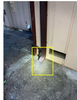
Downspout terminates at foundation
