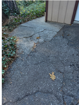
Heavy driveway cracking
