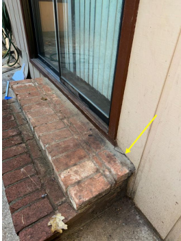
Back side siding to ground contact
