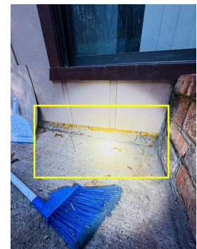
Back left foundation wall spalling/deterioration
