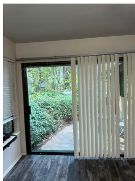
Missing sliding screen door
