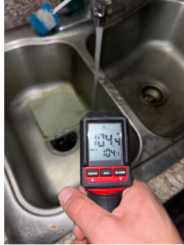
Water temperature noted at 104.4° F
