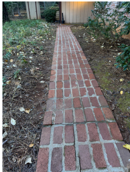
Walkway displacement and trip hazard
