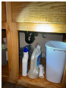
Bathroom 1 blocked sink cabinet
