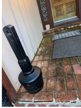
Front siding to ground contact
