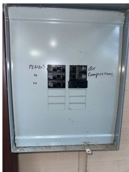
Sub panel 2 detail
