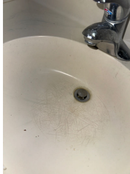
Bathroom 1 cracked sink surface
