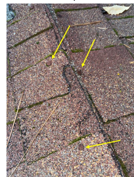
Exposed roof nails
