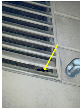
Damaged front left gable end vent screen
