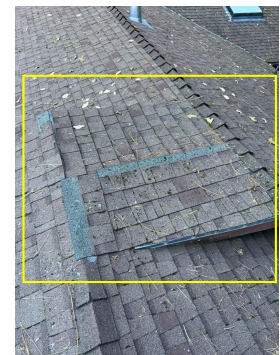
Unprofessional roof installation
