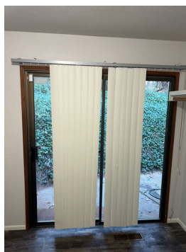
Room 5 missing sliding screen door
