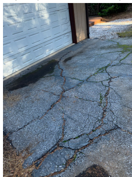
Heavy driveway cracking
