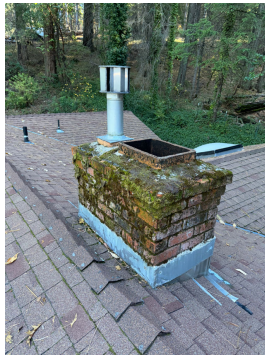
Excessive moss on chimney
