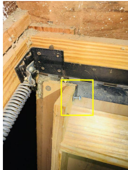
Loose pull down ladder fastener
