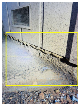
Back left foundation wall spalling/deterioration
