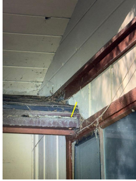
Missing back side kickout flashing
