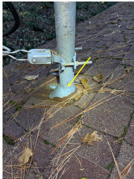
Missing cable feed masthead seal
