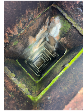
Missing rain cap/spark arrestor
