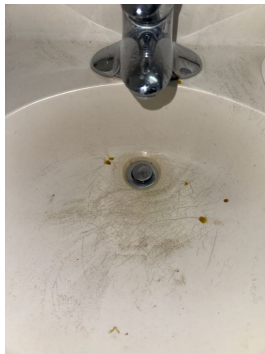
Bathroom 2 cracked sink surface
