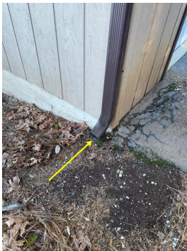
Downspout terminates at foundation
