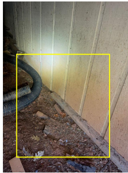
Siding to ground contact
