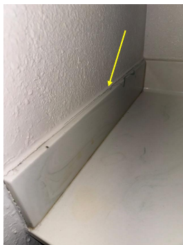
Bathroom 1 deficient counter caulk
