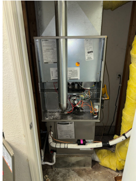
HVAC furnace detail
