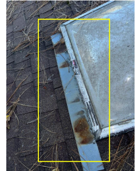
Rusted skylight flashing
