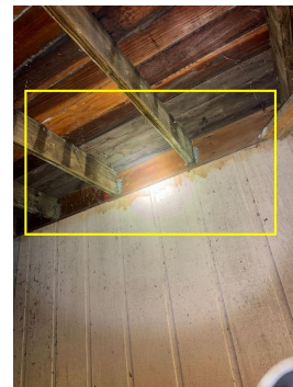
Ledger installed with nails and lacking flashing
