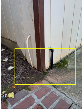
Front side siding to ground contact and decay
