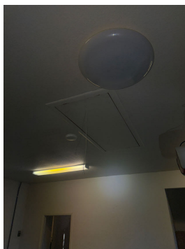
Attic pull down ladder not fire rated
