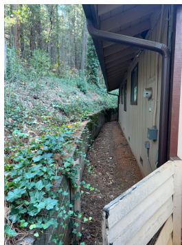
Negative grade toward house
