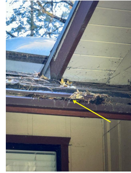
Clogged leafless style gutter guard
