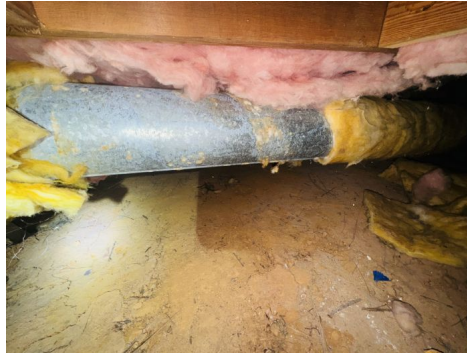
Deficient insulation on ductwork
