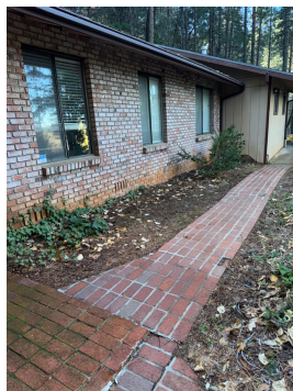
Negative grade toward house
