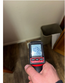
Heating noted at 103.6° F
