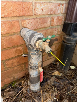
Missing anti siphon vacuum breaker
