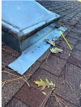
Rusted skylight flashing
