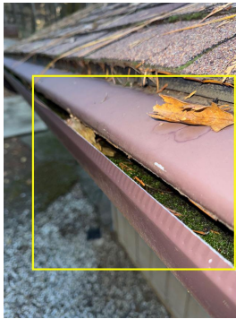
Leafless style gutter guard clogged
