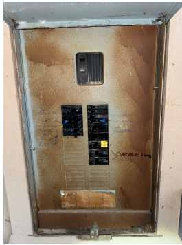
Main service panel detail
