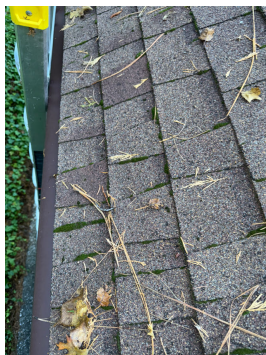
Moss on roof
