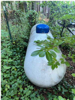
Liquid propane gas tank detail
