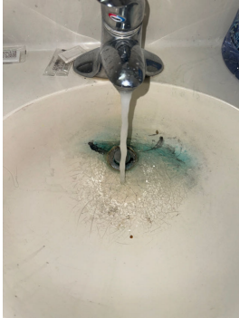
Bathroom 1 cracked and stained sink surface
