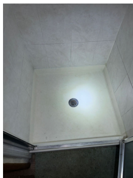
Bathroom 2 stained shower pan
