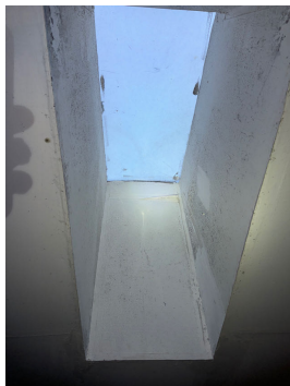
Staining inside skylight
