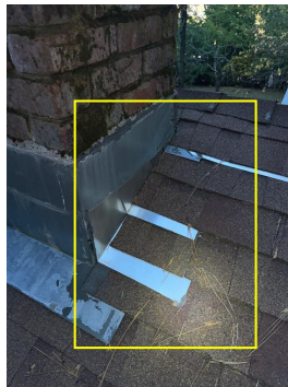
Questionable chimney flashing
