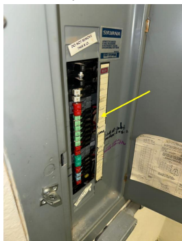
Panel cover not flush against breakers
