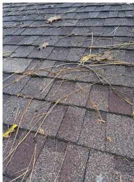
Moss on roof
