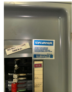
GTE Sylvania brand sub panel
