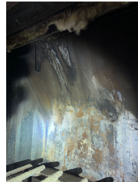
Rust/corrosion inside fireplace
