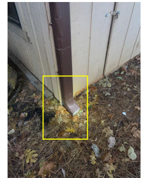
Downspout terminates at foundation
