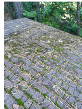
Moss on roof
