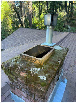
Missing rain cap and spark arrestor
