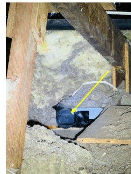
Exhaust vent terminates in attic
