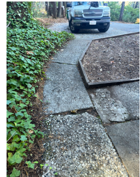
Heavy walkway cracking and displacement
