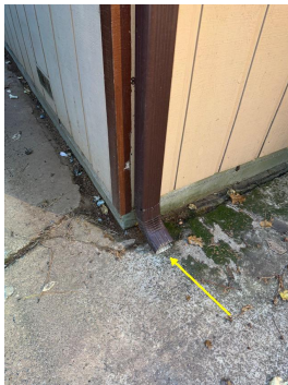
Downspout terminates at foundation
