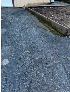
Heavy driveway cracking
