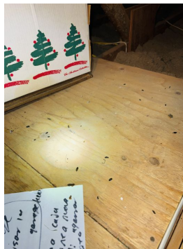
Rodent droppings in attic
