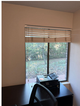
Office window difficult to operate
