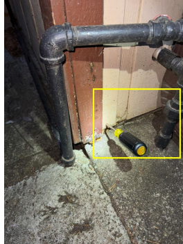
Back side siding decay
