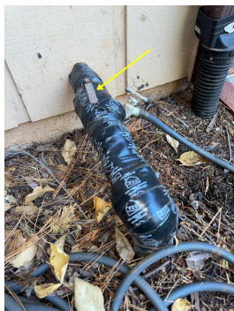
Possible secondary water shut off valve
