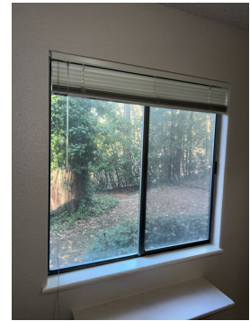
Room 2 possible failed window seal
