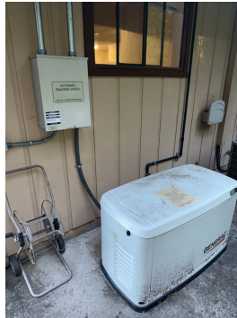
Auxiliary generator system not inspected
