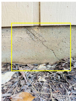
Foundation wall crack
