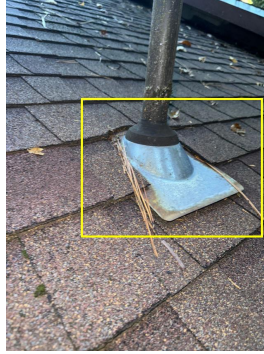
Lifting and rusted flashing
