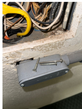
Sharp pointed panel cover screws
