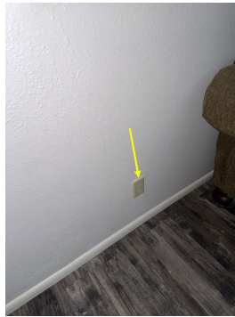
Loose living room outlet
