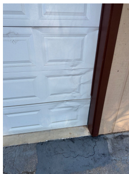
Vehicle door damage
