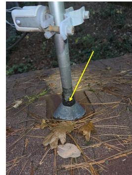
Worn cable feed masthead tape seal
