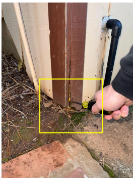
Front side trim to ground contact and decay
