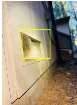
Damaged left side vent screen
