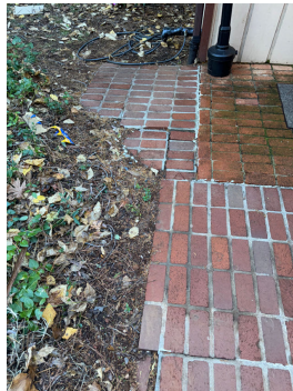
Walkway displacement and trip hazard
