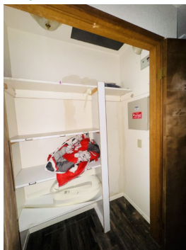
Blocked closet attic access
