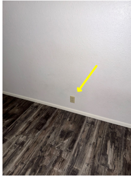
Room 2 loose outlet
