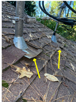
Rusted and lifting flashing
