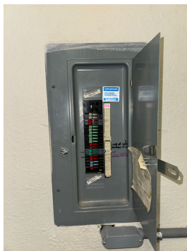
Sub panel detail
