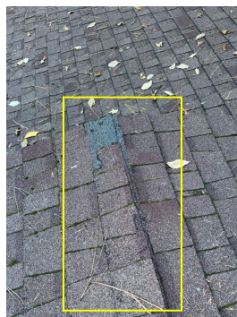
Unprofessional roof installation and/or damage
