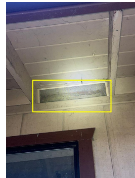
Soffit vent blocked with insulation
