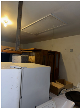
Blocked attic pull down ladder
