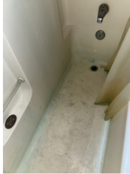
Bathroom 1 stained bathtub
