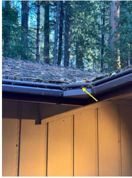
Clogged leafless style gutter guard
