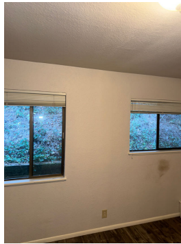
Room 4 possible failed seals
