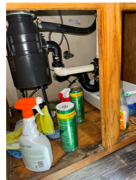
Blocked sink cabinet
