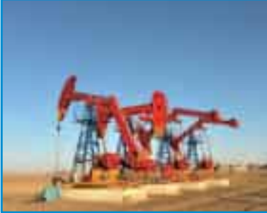
Oil production equipment
