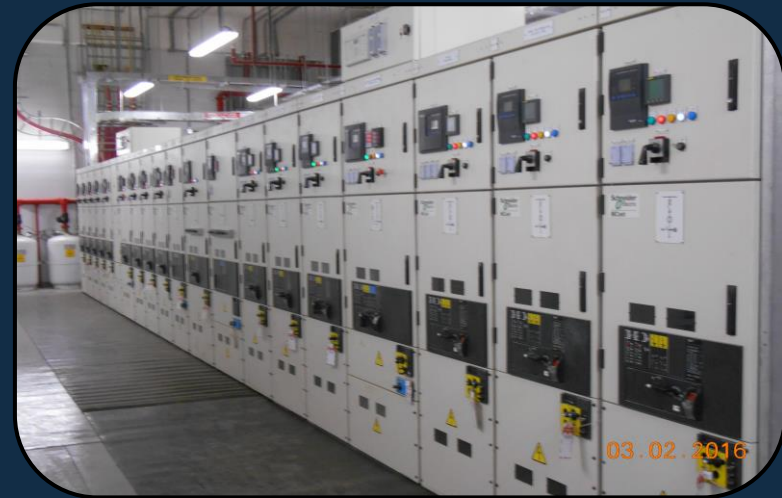
Chillers MV Switchgear (13.8 kV) [Project: King Abdullah Financial District]
