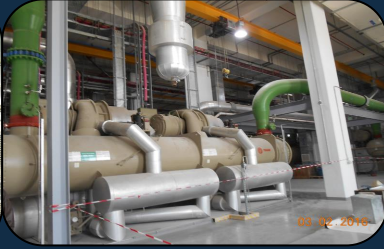
Chilled Water Plant: 6x2,500 Tons water-cooled chillers. Total capacity 15,000 tons. [Project: King Abdullah Financial District]
