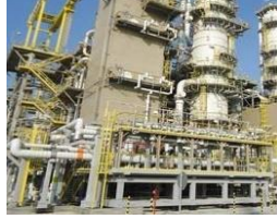
Gas Pre-Treatment and Nitrogen Rejection Units
