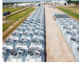
Air Cooled Heat Exchangers
