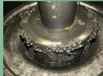
Accumulation of sludge within ECM Pump
