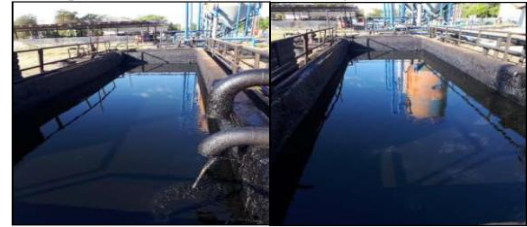
Skimming Tank with 50% level with NX Chemical Treatment
