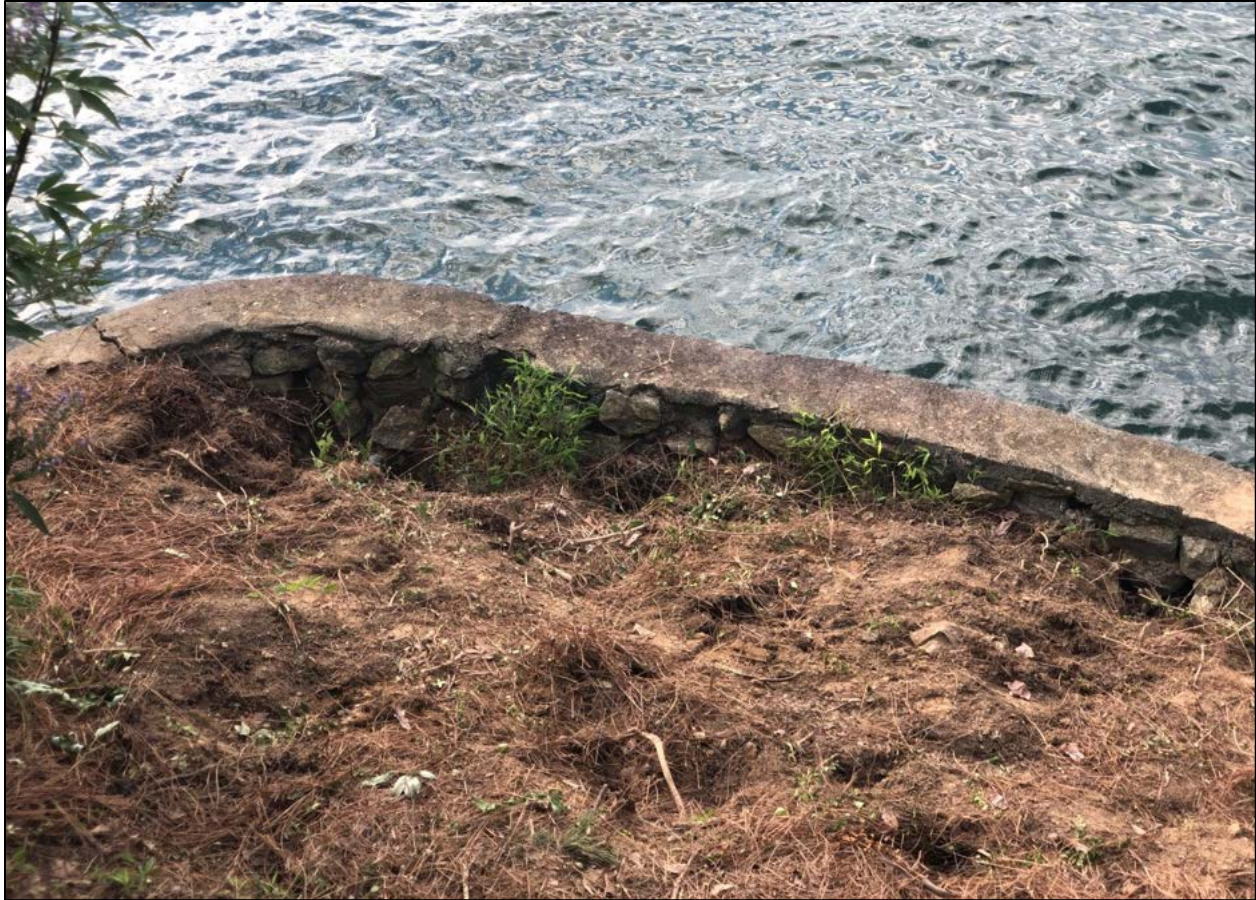
Figure 3-4. Erosion of soils from behind bulkhead on Lake Burton
