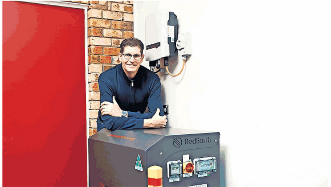
Michael Chard is making a passive income from the solar panel and battery storage system in his home. PHOTO: JAMILA TODERAS
