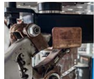
Built-in grounding point
