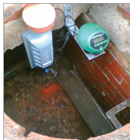
IMP MONITORING IN A CSO CHAMBER
