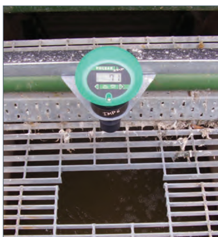
IMP CONTROLLING GATE HEIGHT
