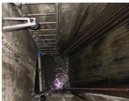
WET WELL 6m WITH LADDER AND FLOAT
