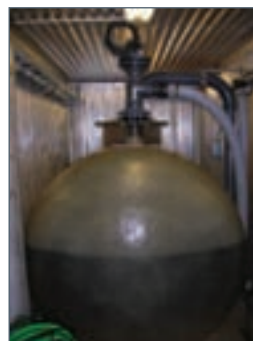
CHEMICAL TANK WITH STANDPIPE 1.9m
