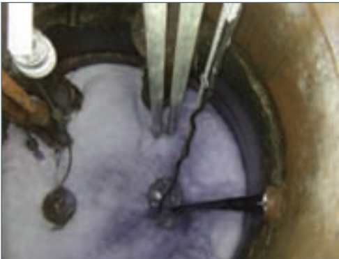
3.5m FOAMY WETWELL PUMP CONTROL
