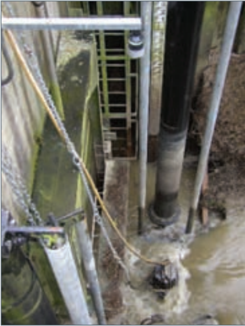
7m PUMP CONTROL
