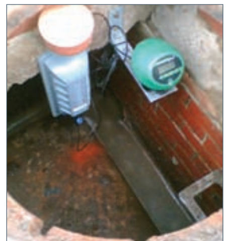
IMP MONITORING IN A CSO CHAMBER
