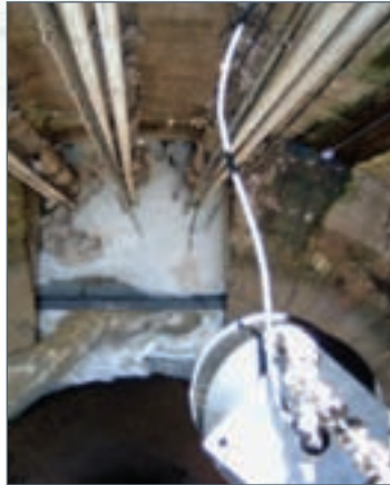
27m STORM TANK 3 PUMPS DOWN CENTRAL WELL
