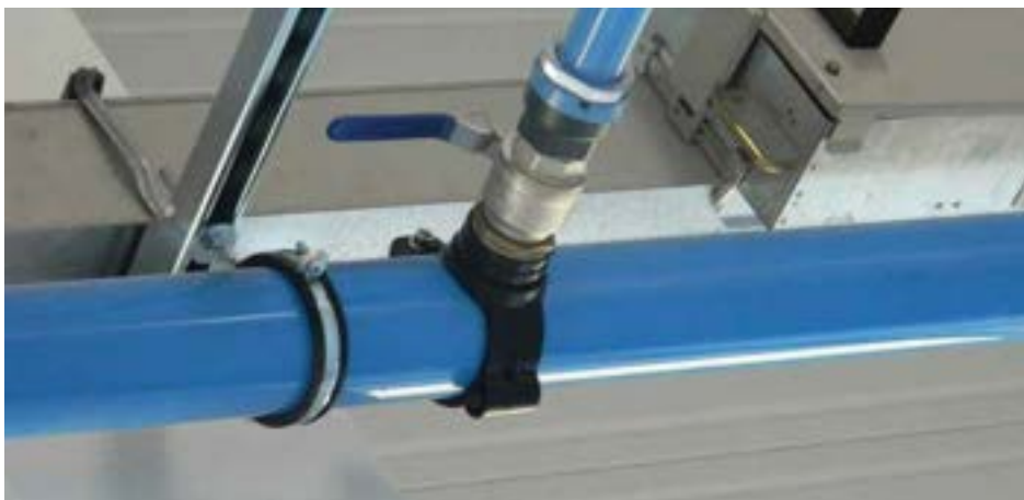
Typical Application for Saddle Branch
