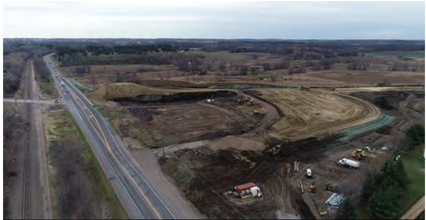
View of the construction area south of Highway 12, where the roadways are being realigned and work on the new bridge has begun.
