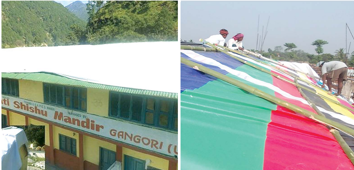
Figure 34. Usage of the Flex Banners to Cover the Leaky Roof of a School [23]
