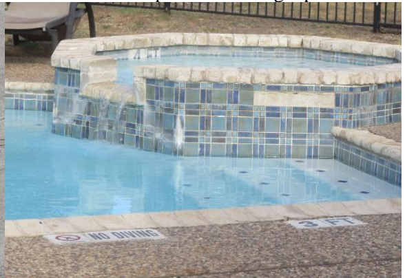
Tiles Missing at the Hill Pool
