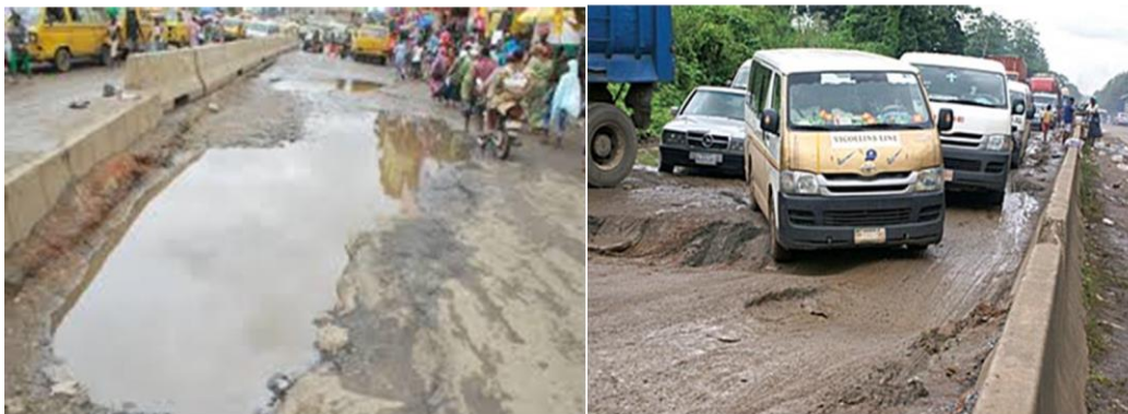
Figure 1. Degenerating Uncompleted and Abandoned Road Projects in the Niger Delta
