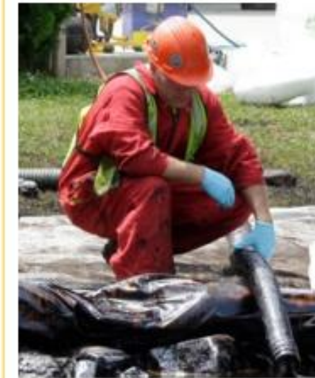
A worker watches water come out of a pipe in Talmadge Creek where booms have been set up to contain an oil spill in Marshall Township, Mich., near the Kalamazoo River. Photo credit: Paul Sancya/ AP/ Shutterstock
