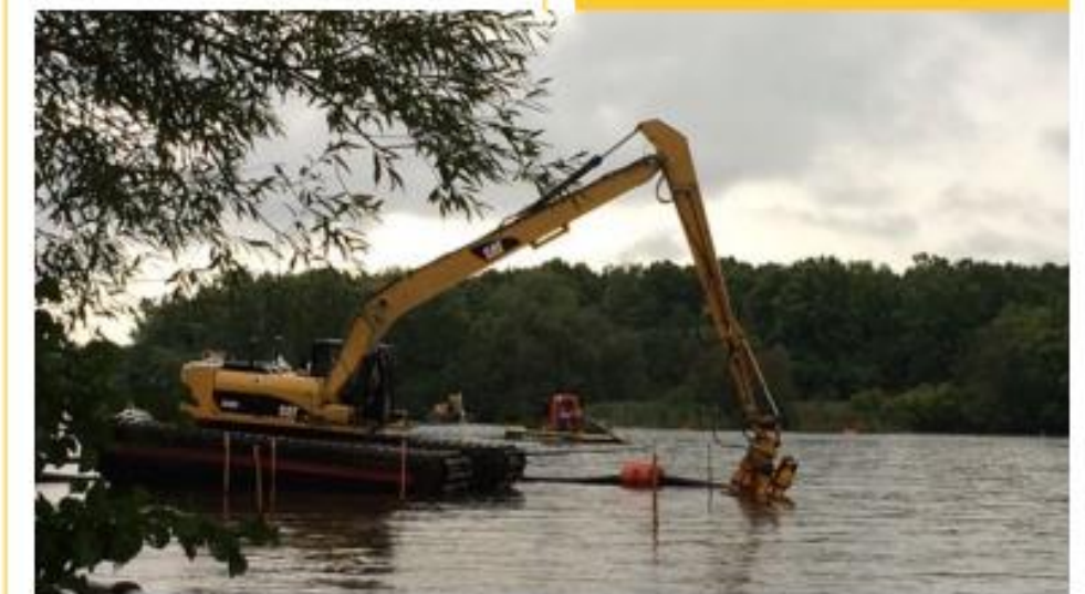
Dredging equipment is utilized to contain and remediate an oil spill near the Kalamazoo River. Photo credit: Justin Ritter.
