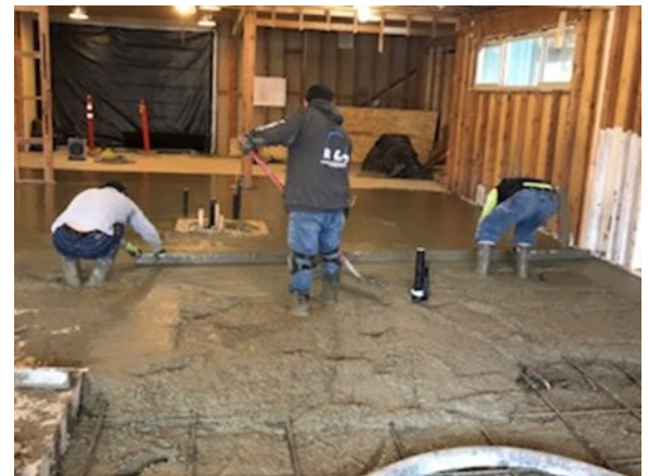
Construction workers pour cement for the new restrooms while Pastor James observes.
