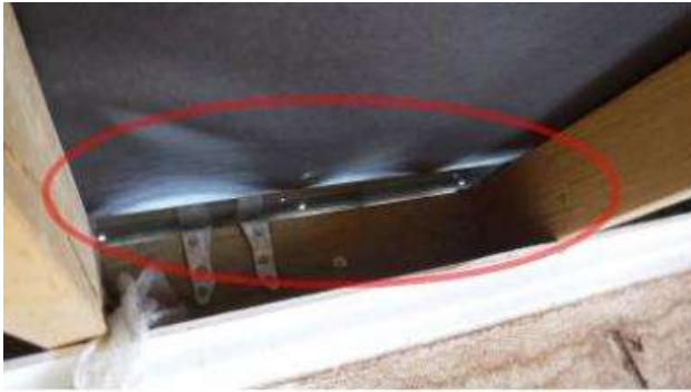
SILLS NOT SEALED / POSSIBLE MOLD AT SILLS.
