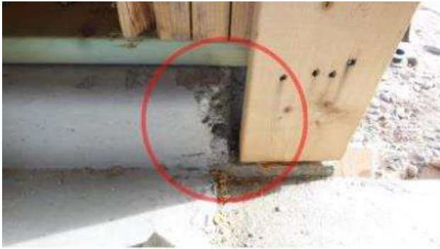
CHIPS IN FOUNDATION AND SLAB.
