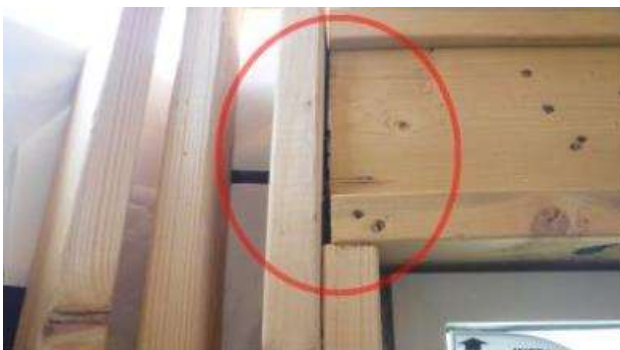
SEPARATIONS AT WINDOW FRAMING.
