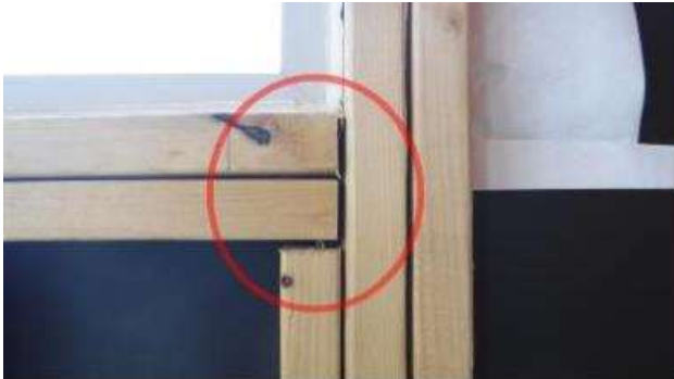
SEPARATIONS AND UNEVEN WINDOW FRAMING.
