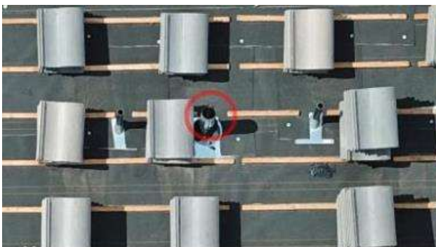
MISSING VENT CAPS AND STORM COLLARS.
