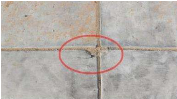
CRACKED-CHIPPED CURB / CONSTRUCTION DEBRIS.
