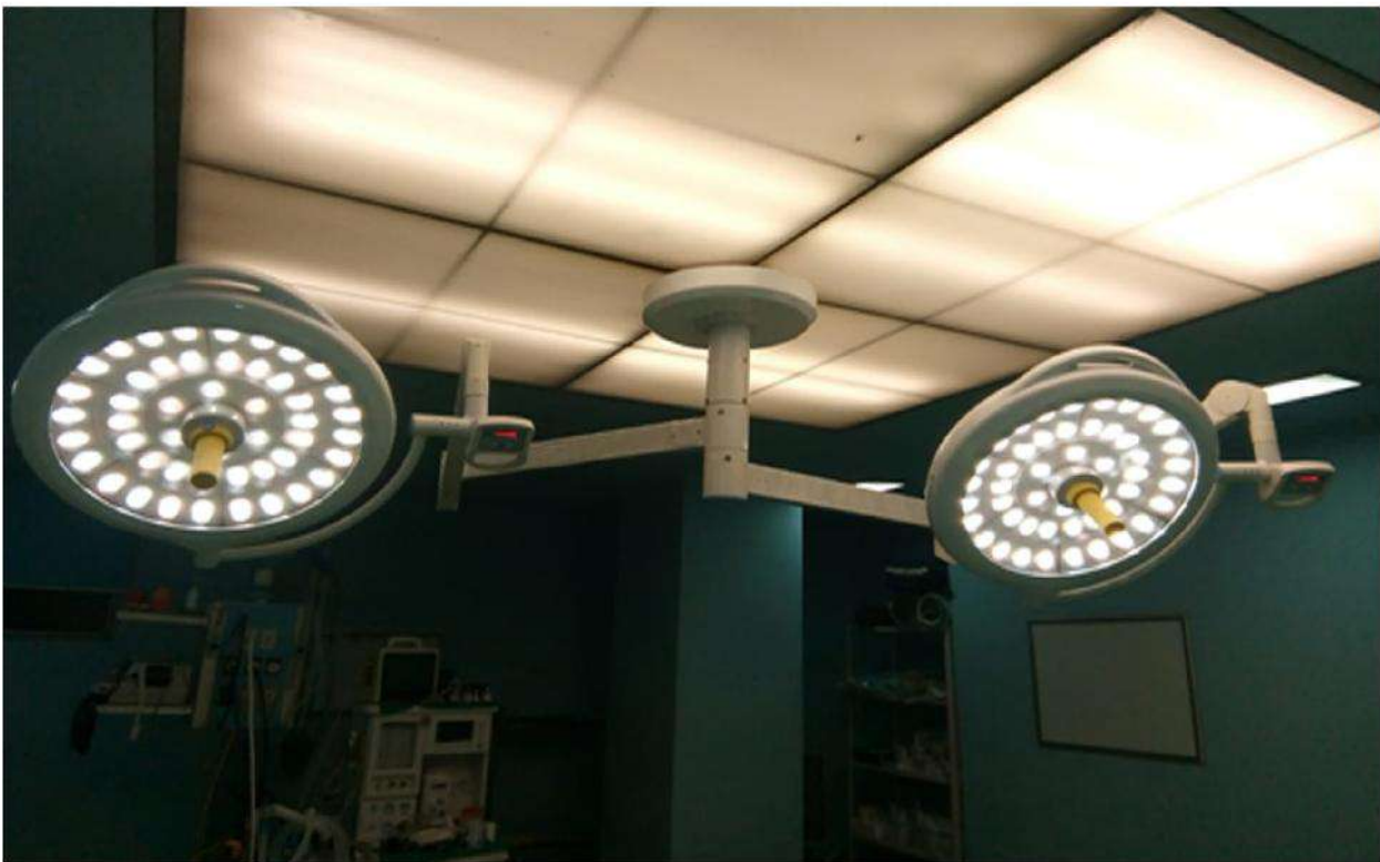
Low Height OT solution where clearance height is between 8ft and 9ft
