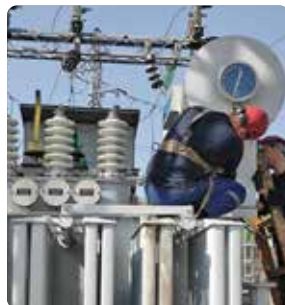
Power Distribution - Installation and Maintenance
