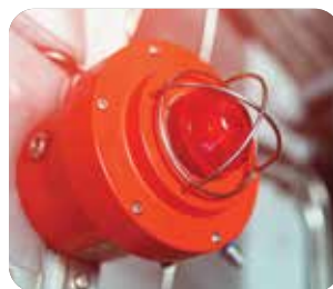
Fire Alarm System
