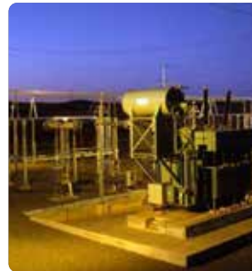
Power upgrade in compliance with DEWA regulations
