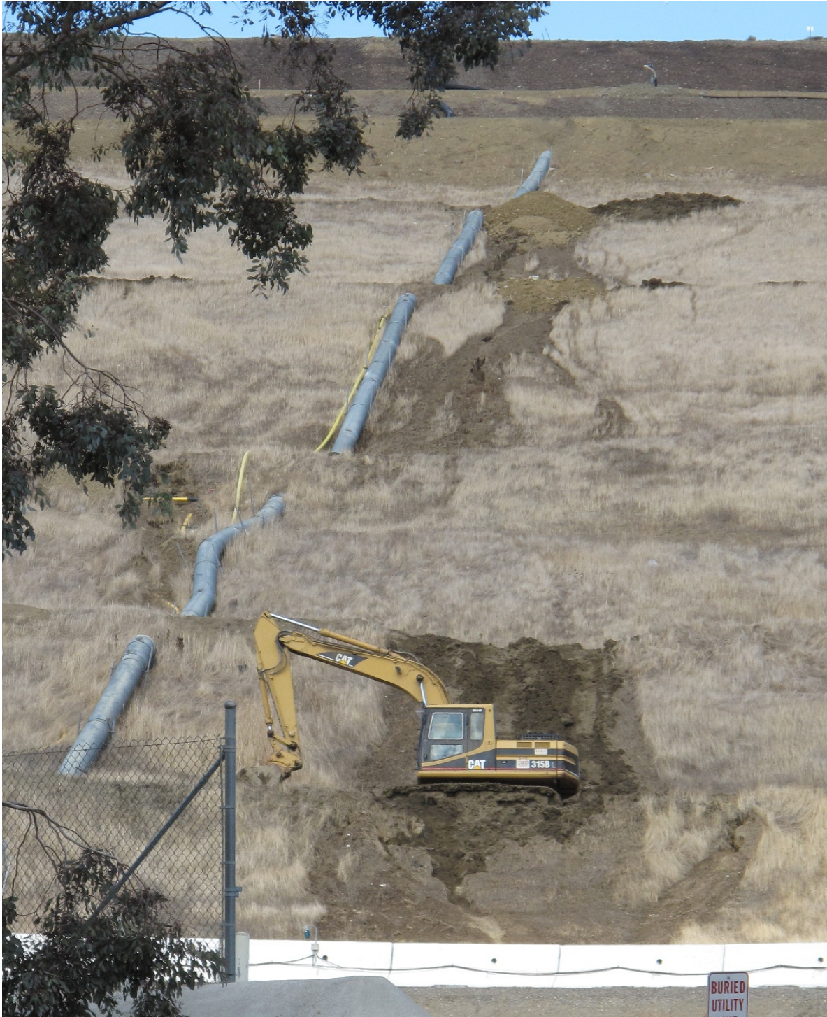
Erosion damage being repaired on front face of closed portion of landfill, from below, looking (approximately) north
