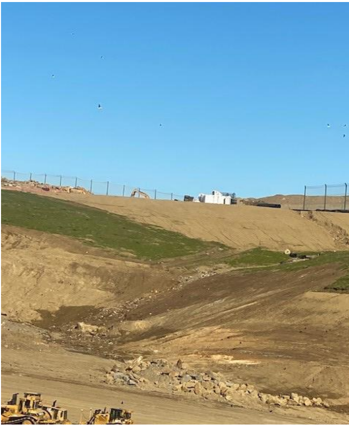
Erosion on the easterly wall, at active phase of FA2.
