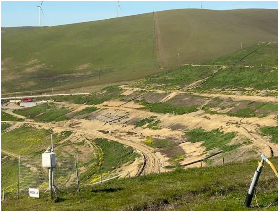
Erosion at ET from storm event, likely December 16, 2022.
