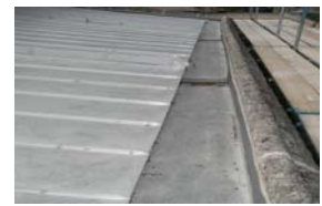
Gutter Lined in Stainless Steel
