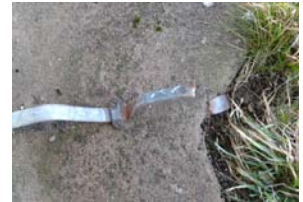
Damaged Lightning Conductor
