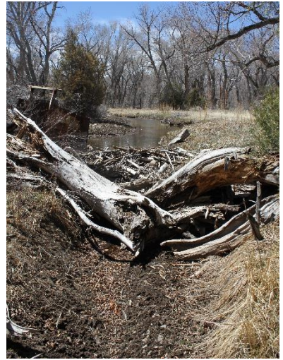
Headgate and feeder ditch looking upstream
