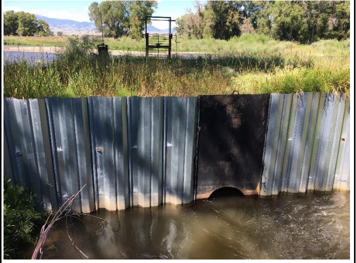
River headgate outlet
