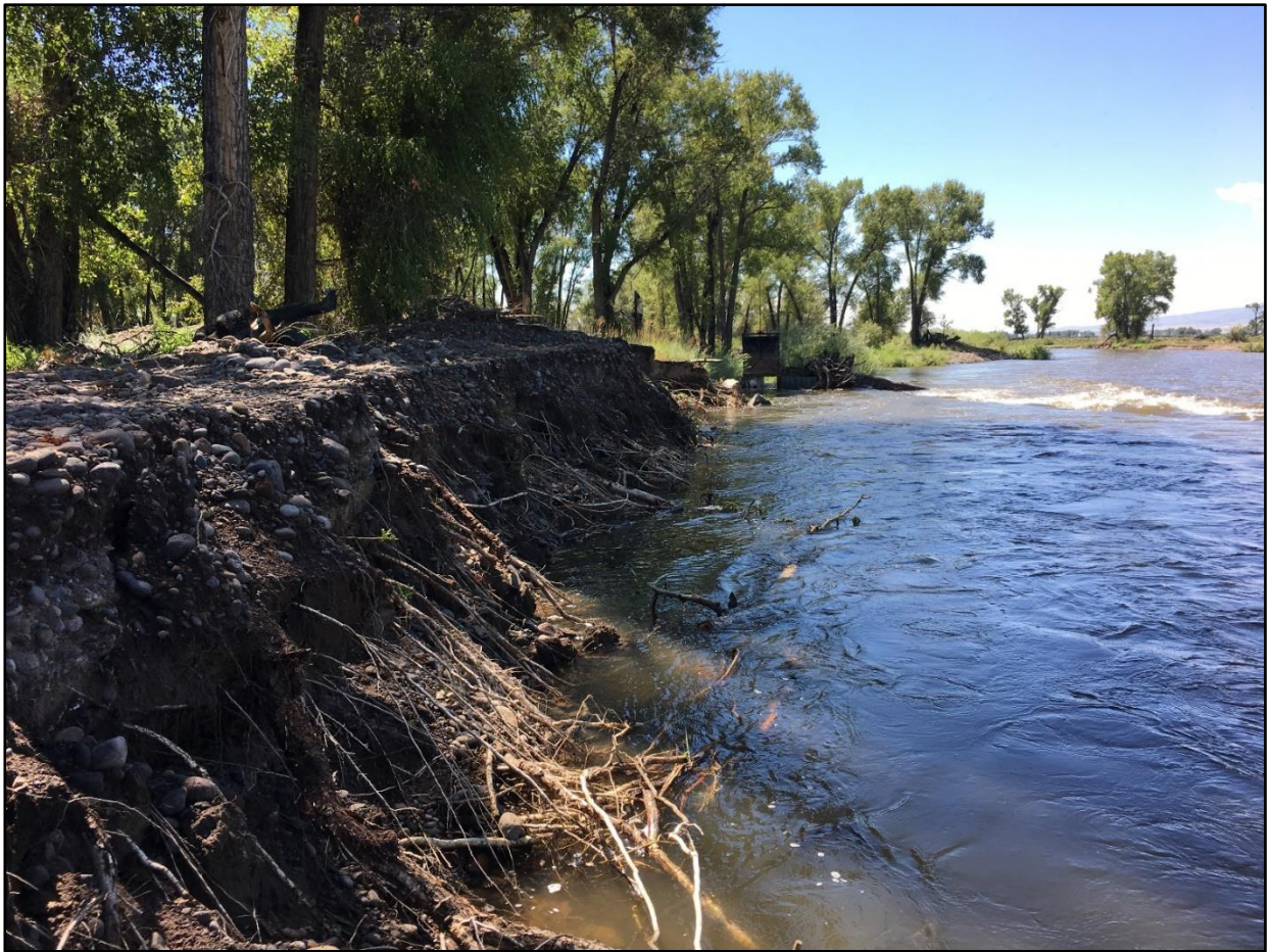
Bank erosion upstream of headgate (north bank)
