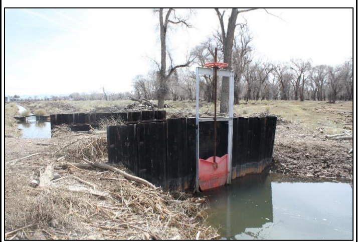
Adjustment headgate outlet
