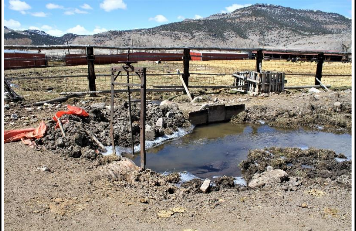
Headgate and overflow gate
