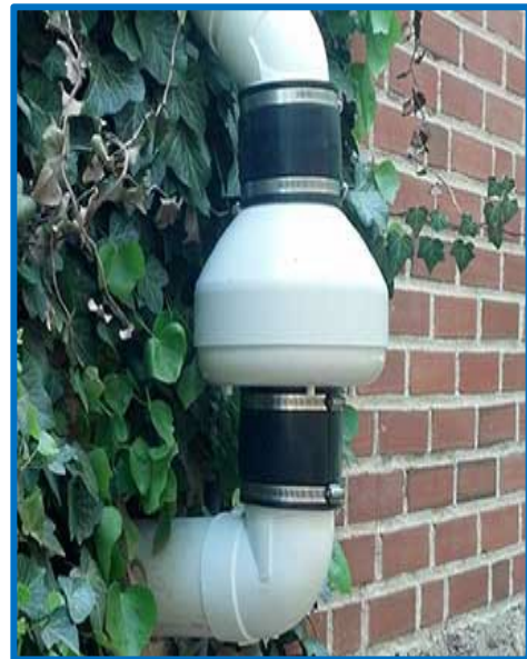
Figure 4.3.10-5 Radon Mitigation Fan Installed on Commercial Building in Martinsburg (SWAT Environmental, 2015)
