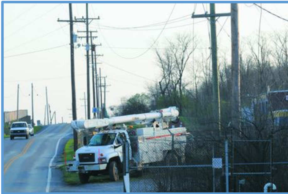
Figure 4.3.23-1 Crew Repairs Damage from Transformer Fire in Berkeley County 3/26/16 (Agnir, 2016)
