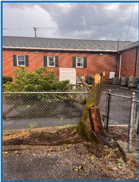
Figure 4.3.11-2: Tree Damage on Burke Street in Martinsburg City, Berkeley County (August 2026).
