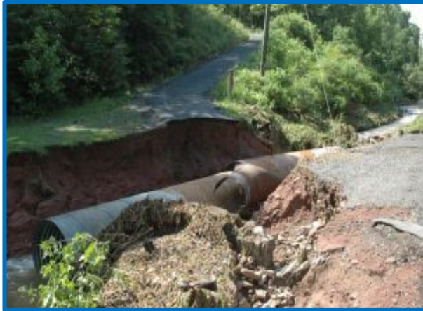
Figure 4.3.8-5: Collapsed Road in Paw Paw (The Morgan Messenger, 2018)
