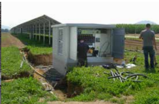
Feed-in joints Solar park
