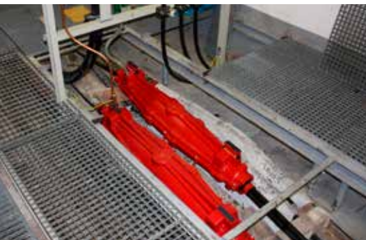
Oil refill joints in switch gear station
