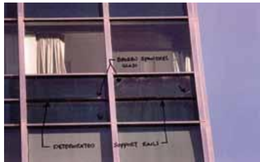
39 Recommended: [39-40] The original windows, which were deteriorated beyond repair, featured a dark tint. They were replaced with a slightly lighter-tinted glazing to improve daylighting in this mid-century modern office building.
