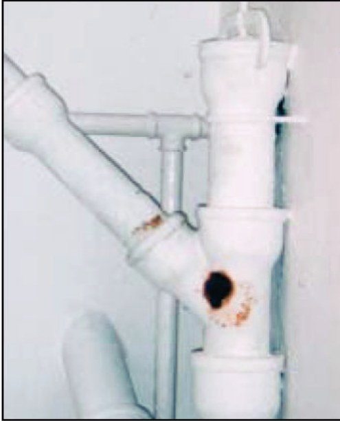
Rust is an indicator that condensation occurs on this drainpipe. The pipe should be insulated to prevent condensation.
