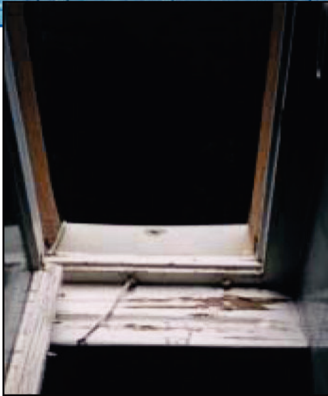
Leaky window – mold is beginning to rot the wooden frame and windowsill.
