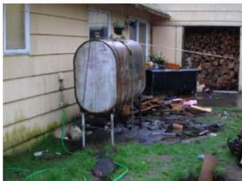
Photo Courtesy of NYSDEC: Oil spill from home heating tank.
