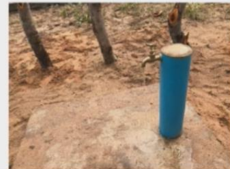
Solar Powered Water Pumps
