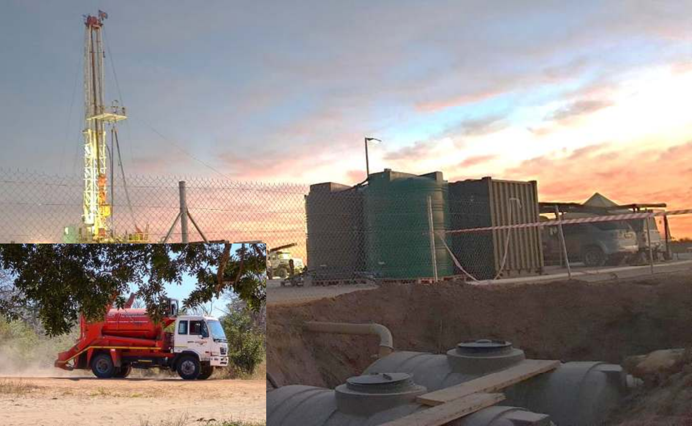
Plate 3.8: Example of the onsite liquid waste management facilities and transfer support to be provided and implemented for each of the proposed drilling locations.
