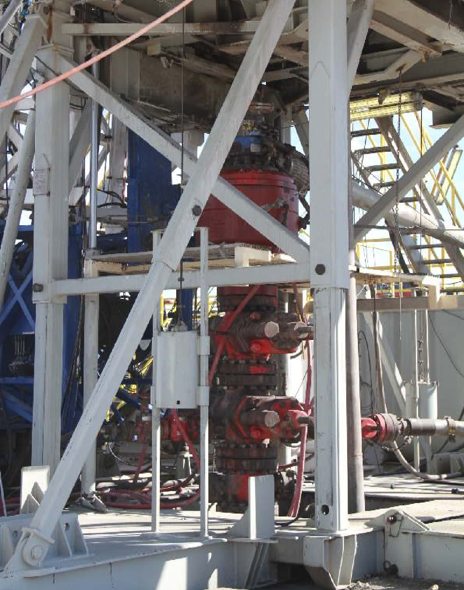
Plate 3.9: The BOP stack to be used in the drilling of multiple exploration and appraisal wells within the AOI in PEL No. 73.
