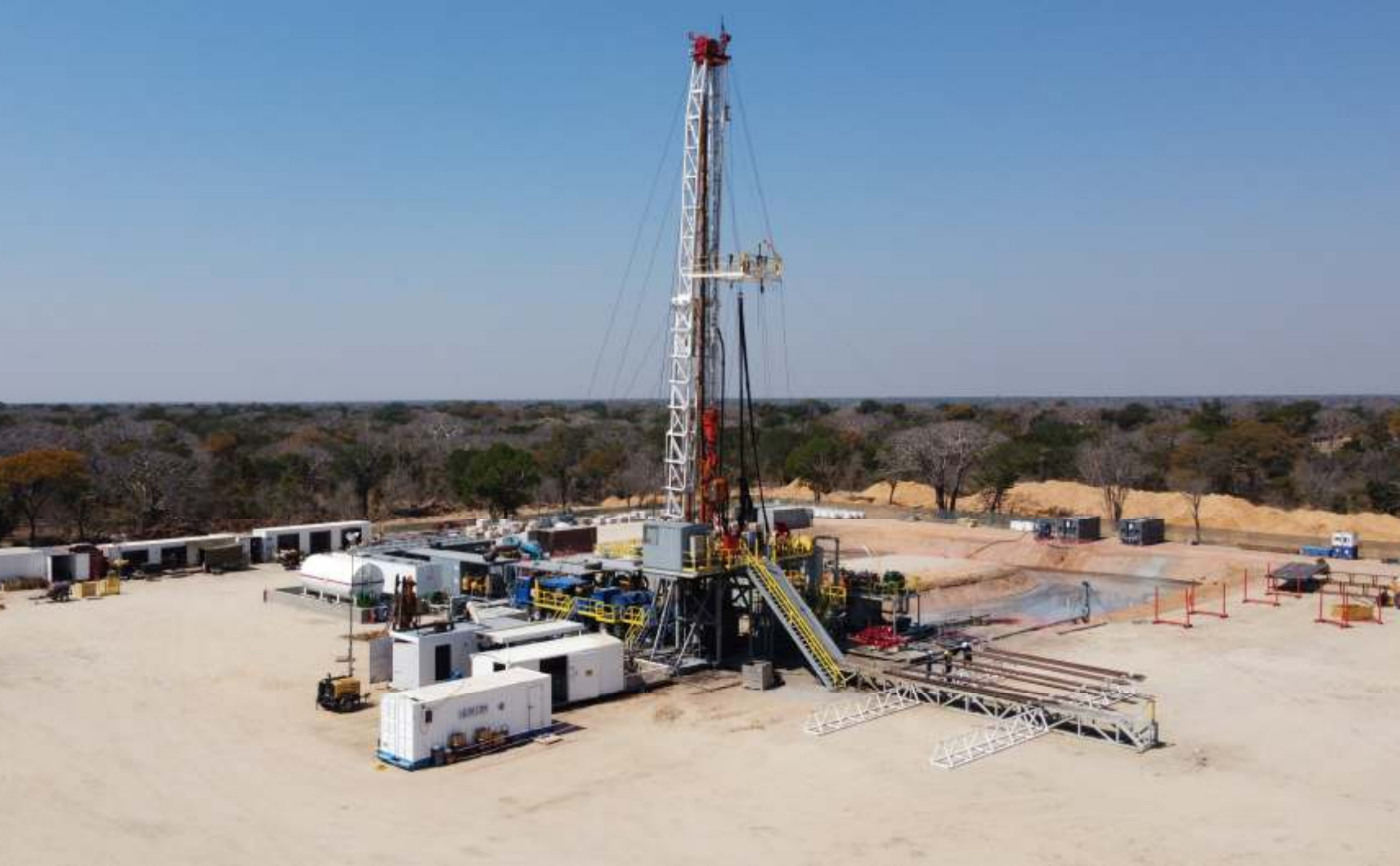
Plate 3.1: The Crown 750 truck mounted drill rig used by REN to drill the stratigraphic wells and will be used to drill the proposed D1-D6 and G1-G6 exploration and appraisal wells in the AOI in PEL No. 73.
