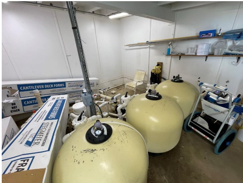
West Cabana - Interior - Pool Equipment
