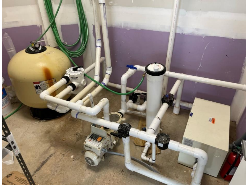
Pump and Filter Equipment
