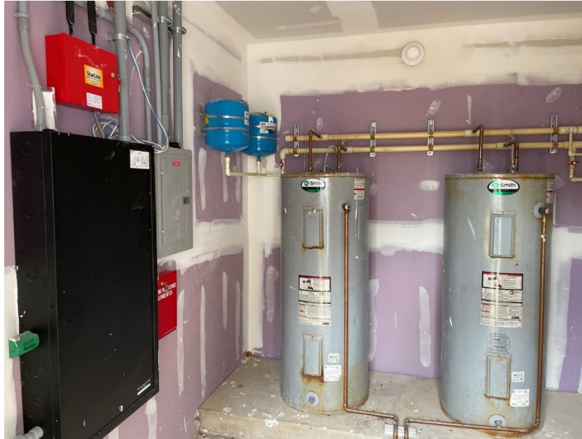
Fire Panel and Water Heaters
