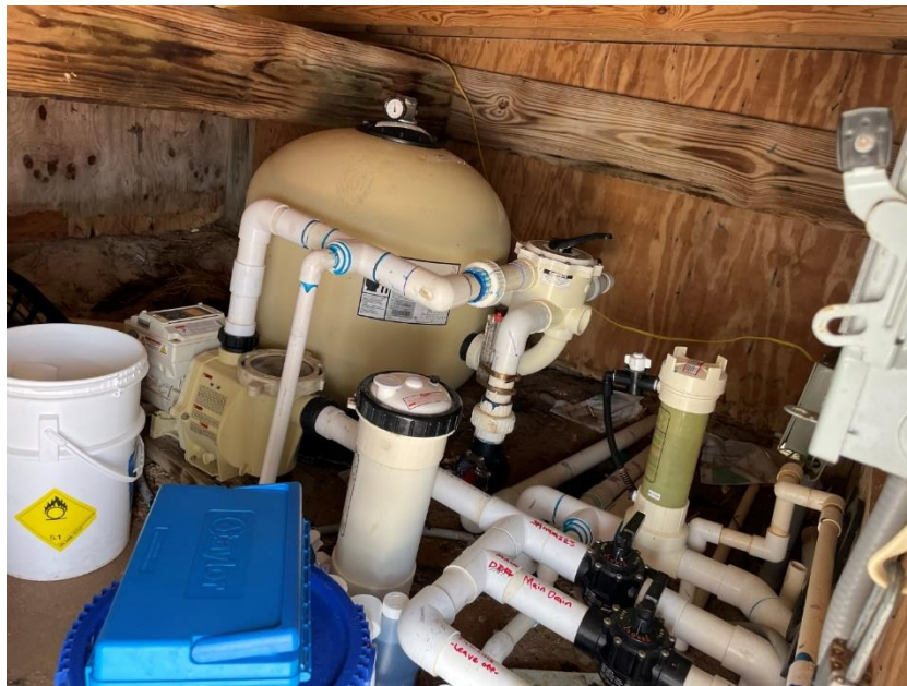
Pump and Filter Equipment – East Pool
