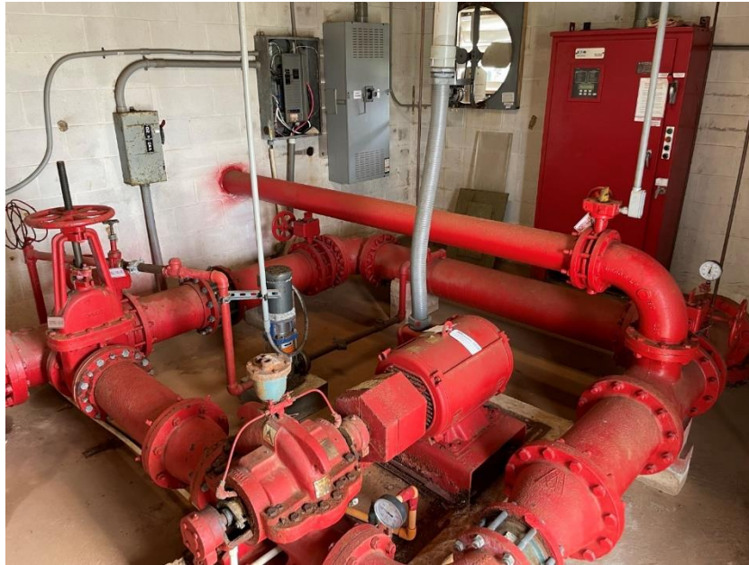
Fire Pump Equipment
