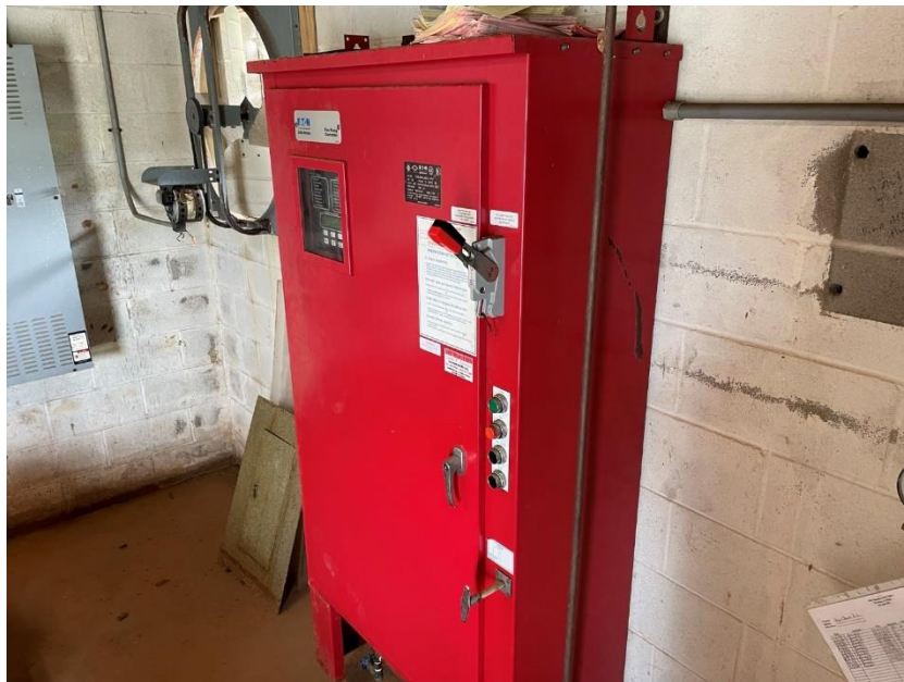
Fire Panel Overview
