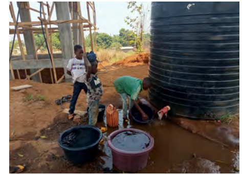
Water from new Tower (background) and Tank (foreground) PREVIEW of Feb 2026
