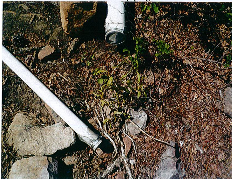
Overflow and drain
