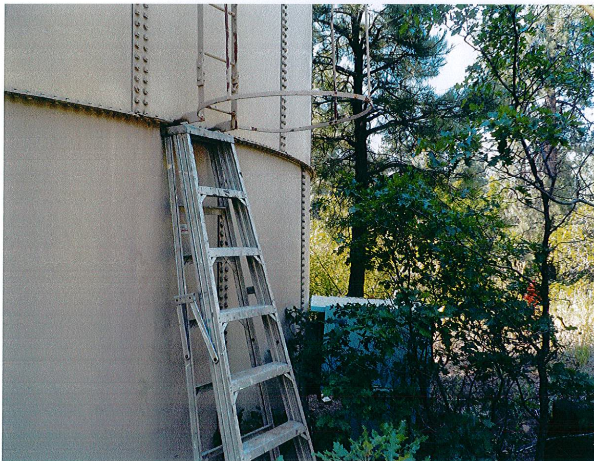
Exterior paint condition is good on the shell surface. Observed spot area's of light surface rust and peeling paint on the upper ring wall, next to the ladder.
