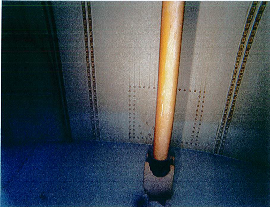
The overflow is PVC, piped thru the bolted shell
