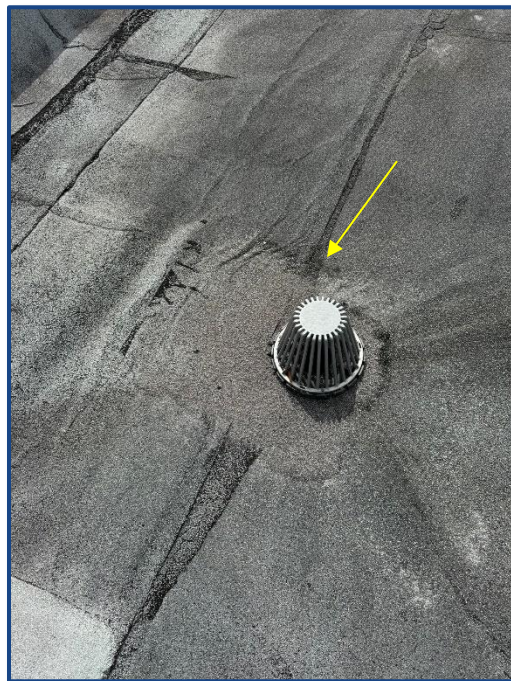
Photograph No. 30: Debris buildup near roof drain.
