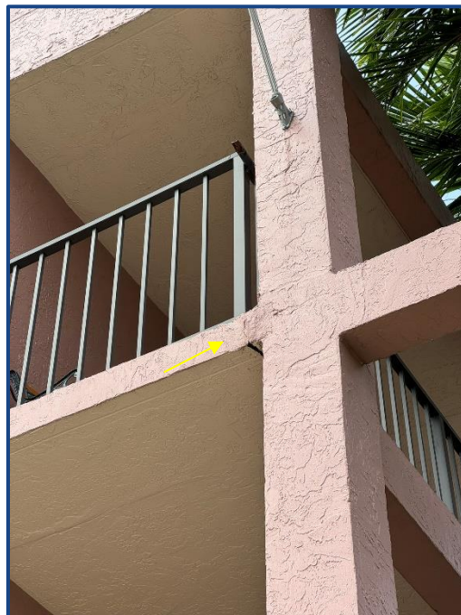
Photograph No. 10: Deteriorated expansion joint observed at 3 rd floor near elevator.
