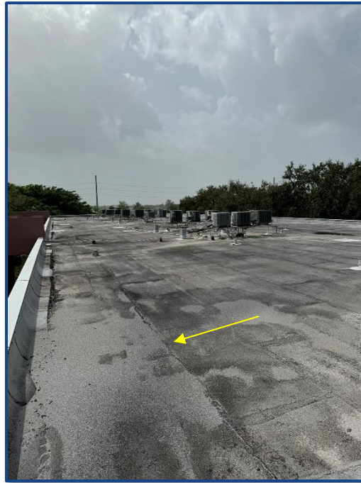
Photograph No. 31: Debris buildup from previous ponding water observed.
