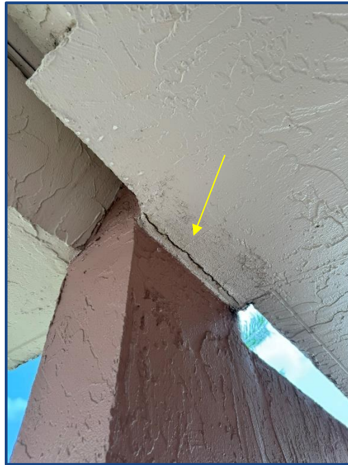
Photograph No. 11: Deteriorated expansion joint observed at 3 rd floor near elevator.
