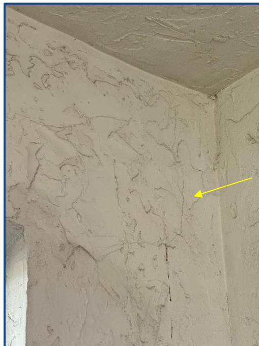
Photograph No. 24: Unit 101: Wall cracking observed near unit sliding glass door.
