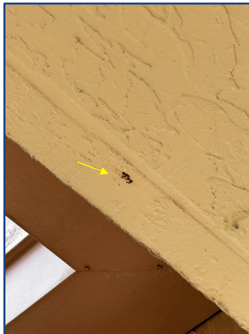
Photograph No. 18: Rust spot observed overhead near unit 310.
