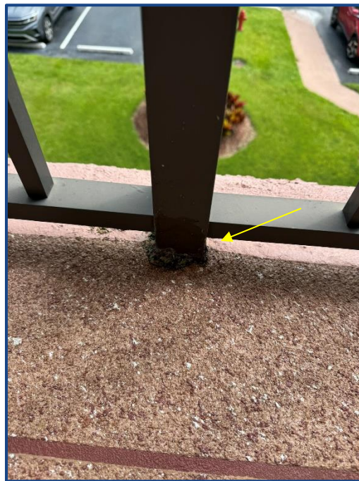
Photograph No. 16: Deteriorated railing post pocket observed near unit 310.
