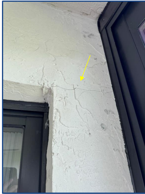
Photograph No. 19: Unit 108: Wall cracking observed near unit sliding glass door.
