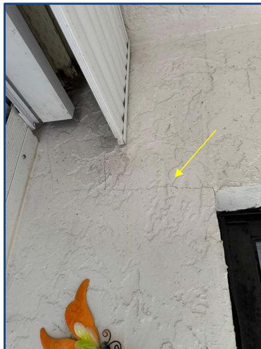
Photograph No. 22: Unit 103: Wall cracking observed near unit sliding glass door..
