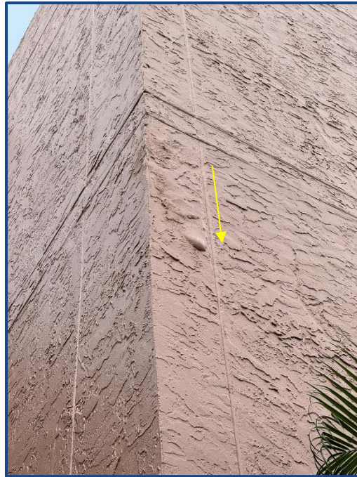
Photograph No. 9: Blistering paint observed at building edge.
