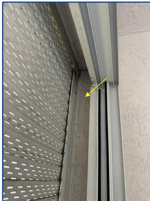
Photograph No. 26: Unit 205: Wall cracking observed near balcony enclosure.
