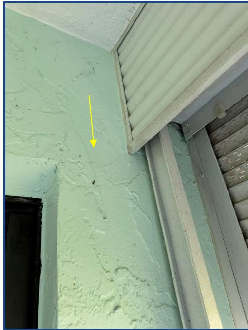
Photograph No. 21: Unit 104: Wall cracking observed near unit sliding glass door.
