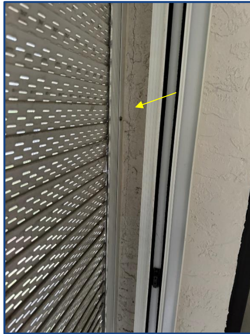
Photograph No. 25: Unit 205: Wall cracking observed near balcony enclosure.
