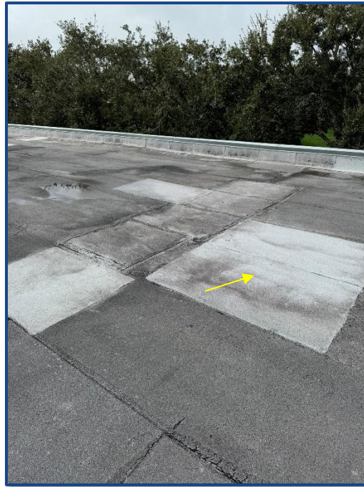
Photograph No. 29: Previous roofing repairs observed at the roof.
