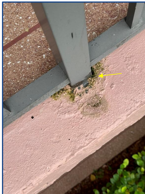
Photograph No. 12: Deteriorated railing post pocket observed near unit 208.
