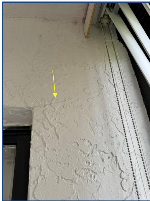
Photograph No. 20: Unit 106: Wall cracking observed near unit sliding glass door.
