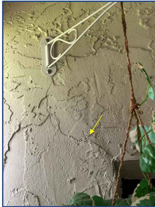
Photograph No. 23: Unit 101: Wall cracking observed near unit sliding glass door.
