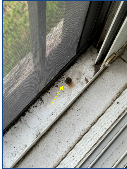
Photograph No. 27: Unit 205: Deteriorated fasteners observed at aluminum enclosure bottom rail.
