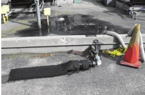
EVAC Filters from concrete containment
