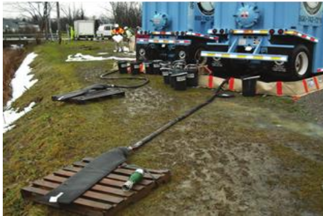
EVAC Filters used to filter water from fac tank
