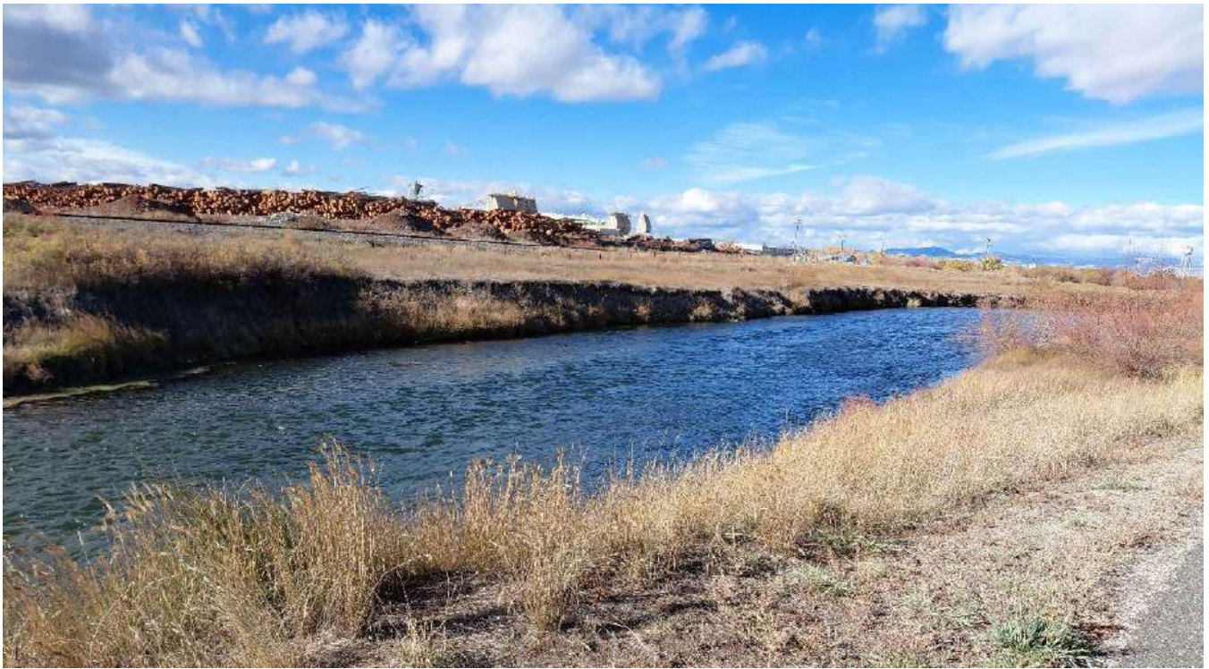
Streambank erosion near Arrowstone Park
